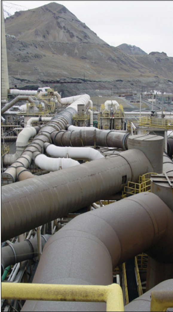
Retrofits to Fume Filtration System at precious metals smelter cuts use of compressed air by nearly 70%.
