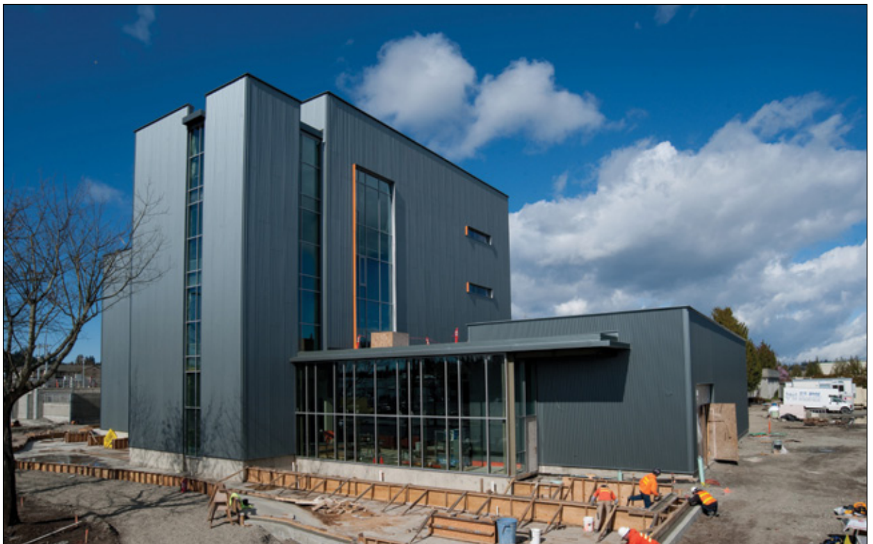
The new cogeneration system supports plans to earn LEED Certification for the LOTT Regional Services Center.
