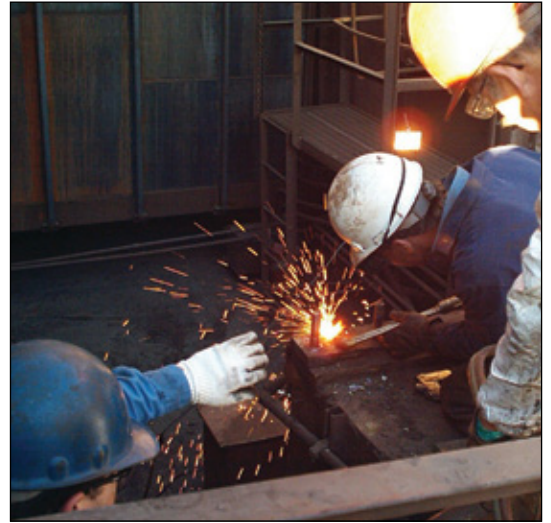
Crews at Oregon-based steel mill prepare for installation of new energy-efficient material handling system.
