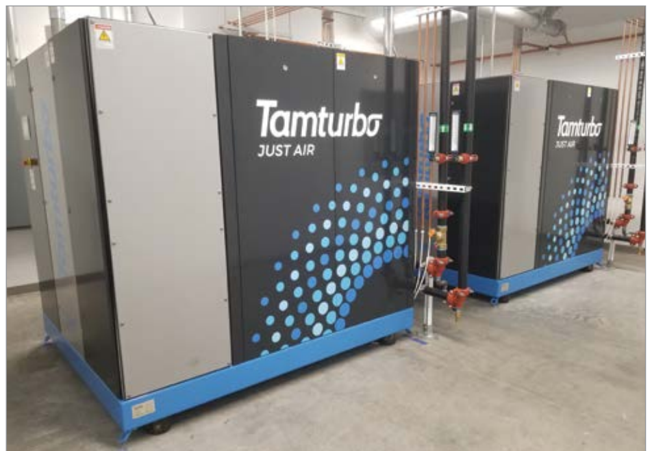
One air compressor as standby/backup. This unit is 100% oil free, with very low maintenance and variable speed drive.
