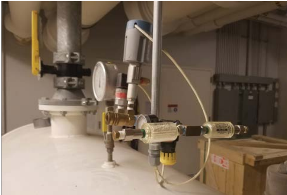
Adding mechanical oil and water indicators on the dry tanks added further assurance of air quality.
