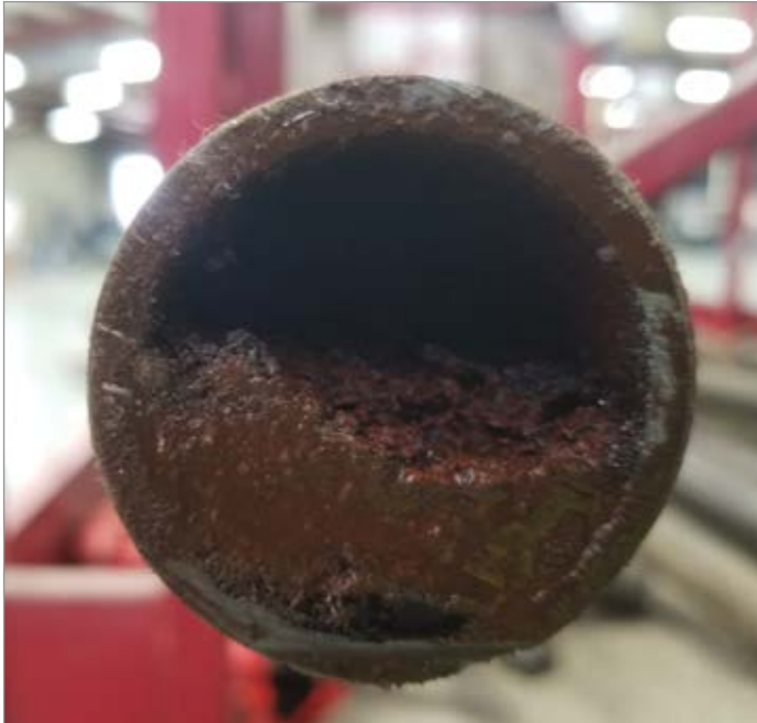
Rust and particle fallout from black pipe in air compressor system.
