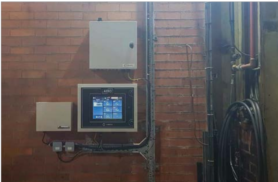
The AERO command and control unit is locally installed and digitally connected via the cloud.
