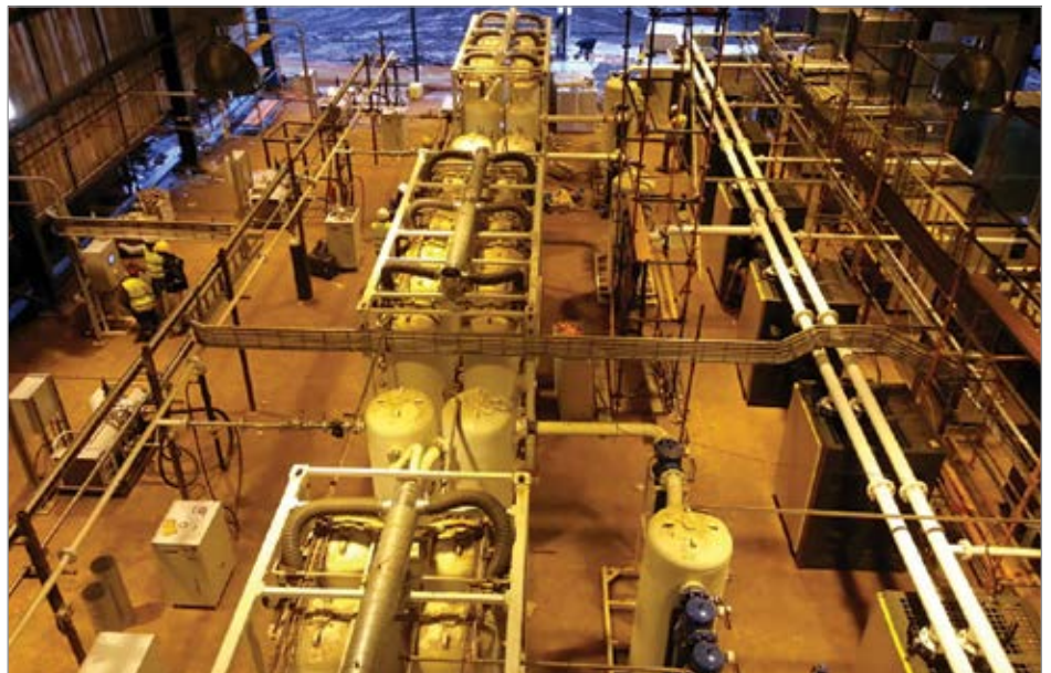
Oxygen production with PSA plants in an African gold mine, on the left in the picture a HAUG.Sirius oxygen compressor. (© HAUG Sauer Kompressoren AG)
