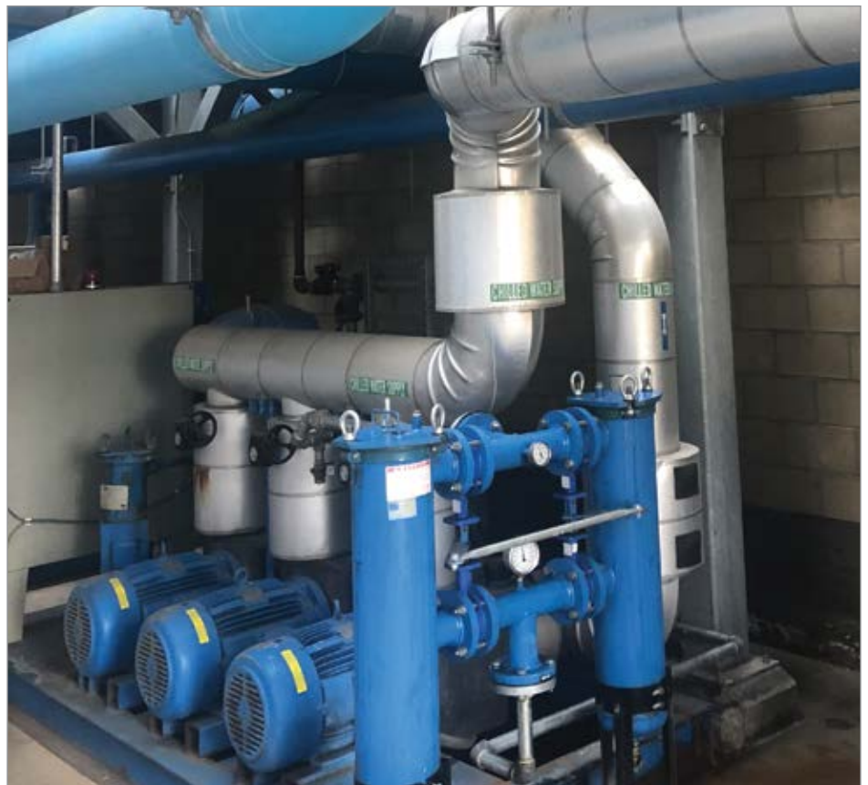
A pump skid for a chilled water system.
