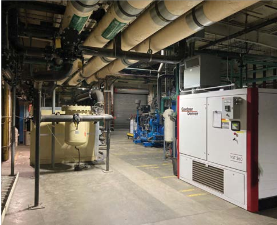
An air compressor room with water-cooled centrifugal and variable-speed rotary screw air compressors.
