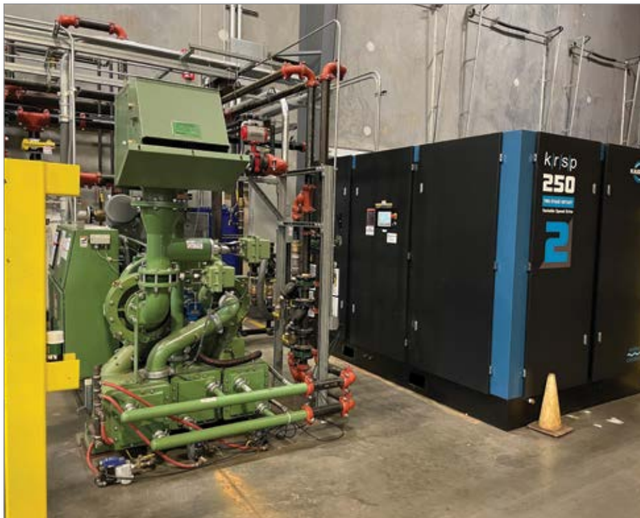
An air compressor room with centrifugal and two-stage rotary screw air compressors.
