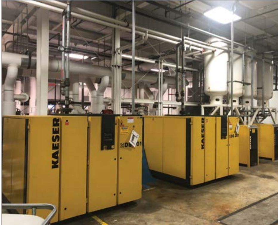
An air compressor room with single-stage rotary screw air compressors and refrigerated compressed air dryers.
