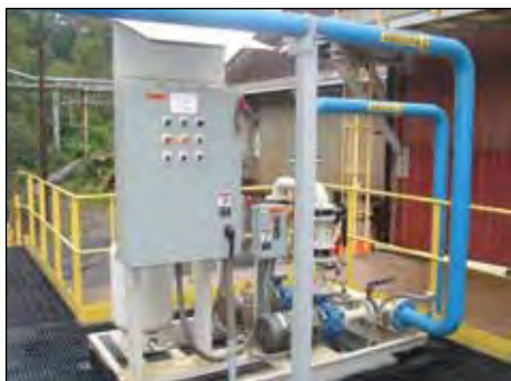
Closed Loop Dual Pump Station and Controller
