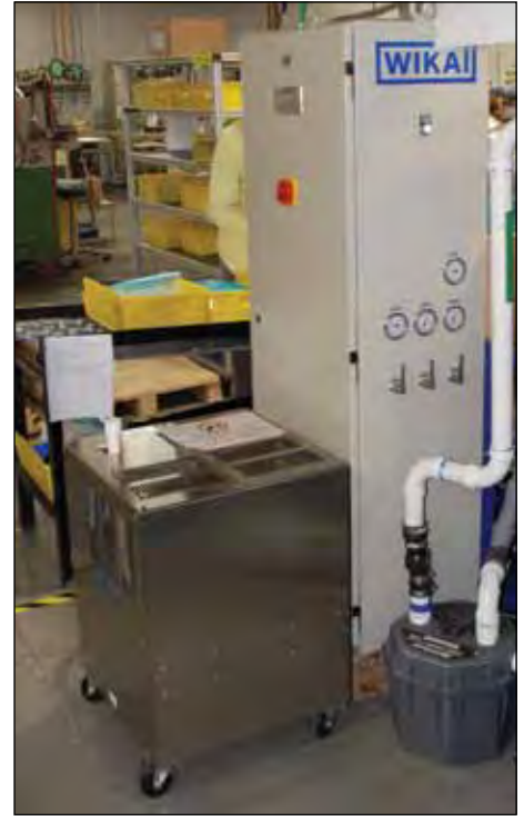
Chillers Reduced Water Consumption at WIKAI
