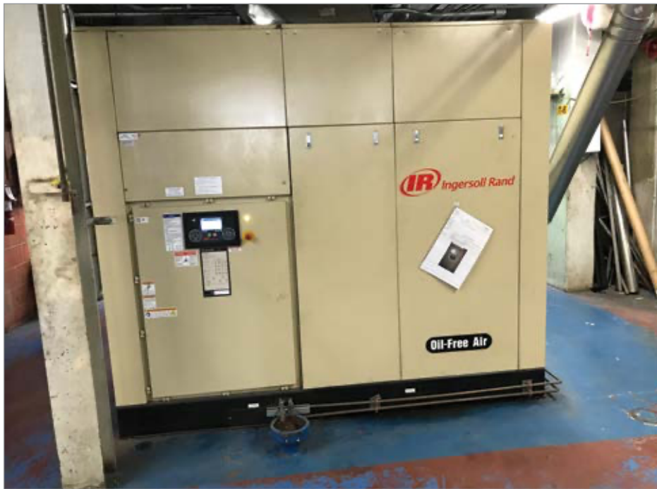
An oil-free rotary screw air compressor at the Molson Coors Toronto Brewery.
