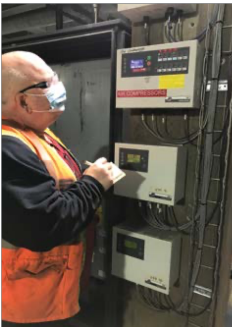
Dino DeFilippis, from Airergy Management Services, monitors air compressor energy consumption.
