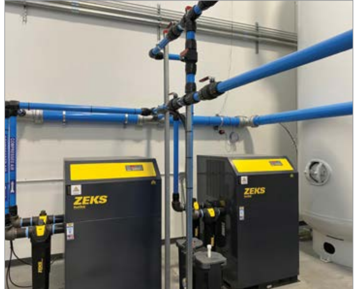
The Delavan compressed air system is designed identically with two refrigerated cycling dryers and other key components for full redundancy. (Photo courtesy of Schoeneck Containers, Inc.)
