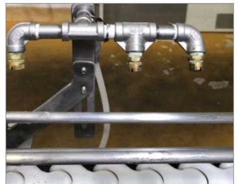
Three brass nozzles designed for spraying liquid being used improperly to blow air on a food packaging line.
