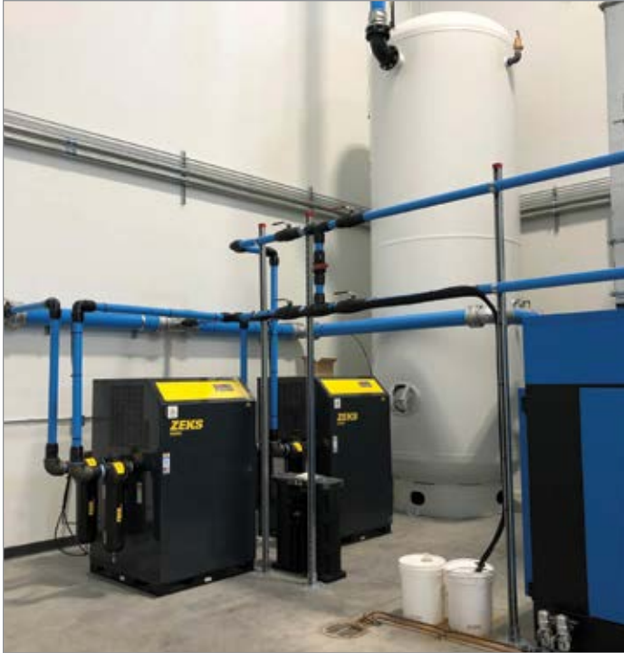
The compressed air system at SCI's Delavan plant includes a 3,800-gallon dry receiver tank. (Photo courtesy of Zorn Compressor & Equipment)
