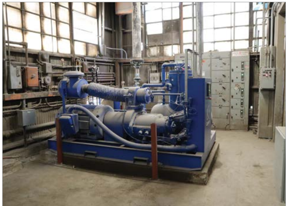
Rotary screw air compressors are used to power a wide variety of applications at CalPortland cement and ready mix plants.
