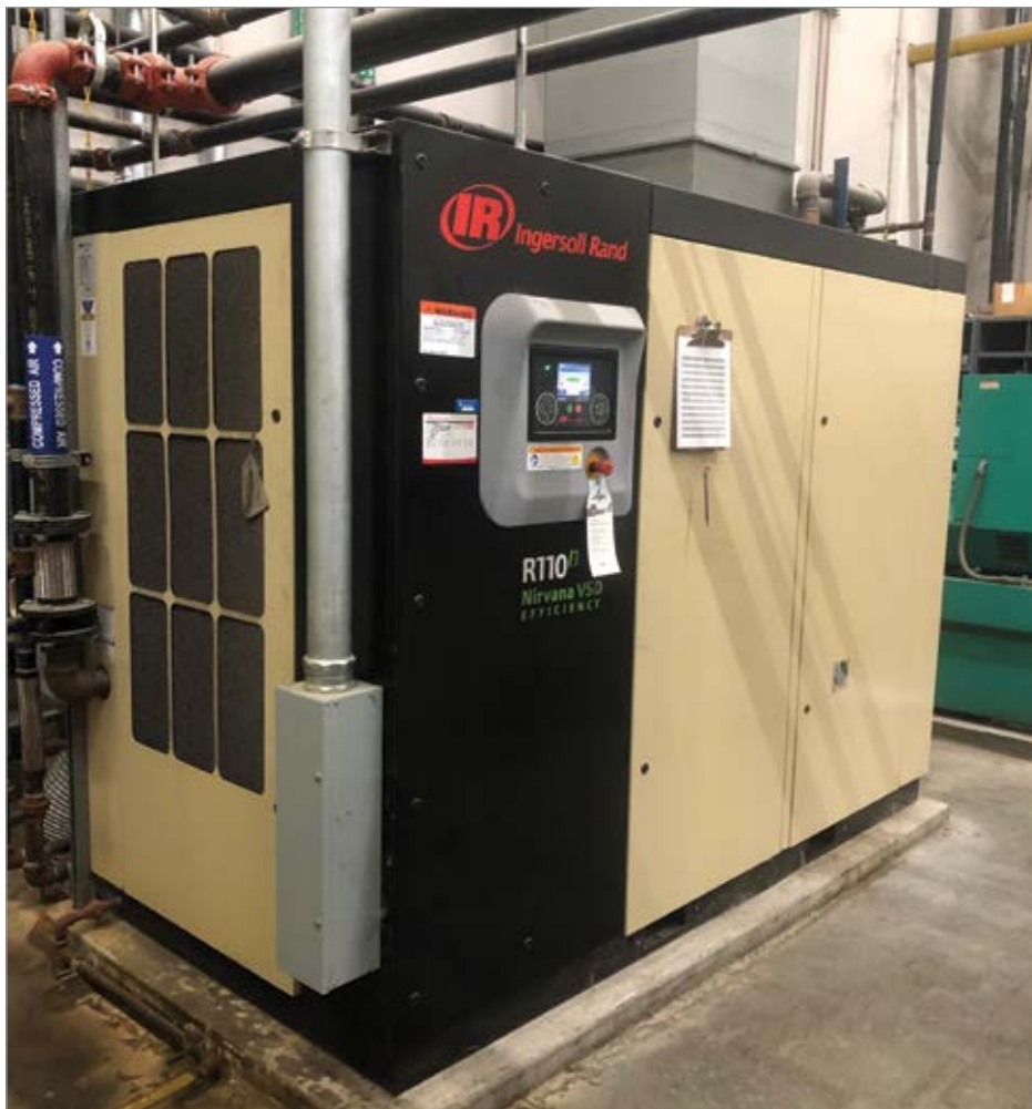
The rotary screw air compressor installed at the Carbondale, Illinois plant.
