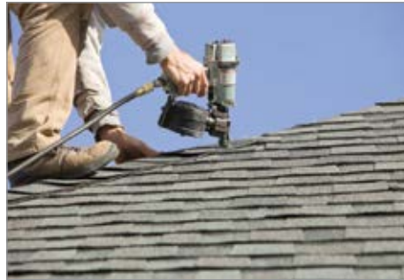
Roofer using an efficient pneumatic nail gun operating from a small gasoline powered or electric powered air compressor.
