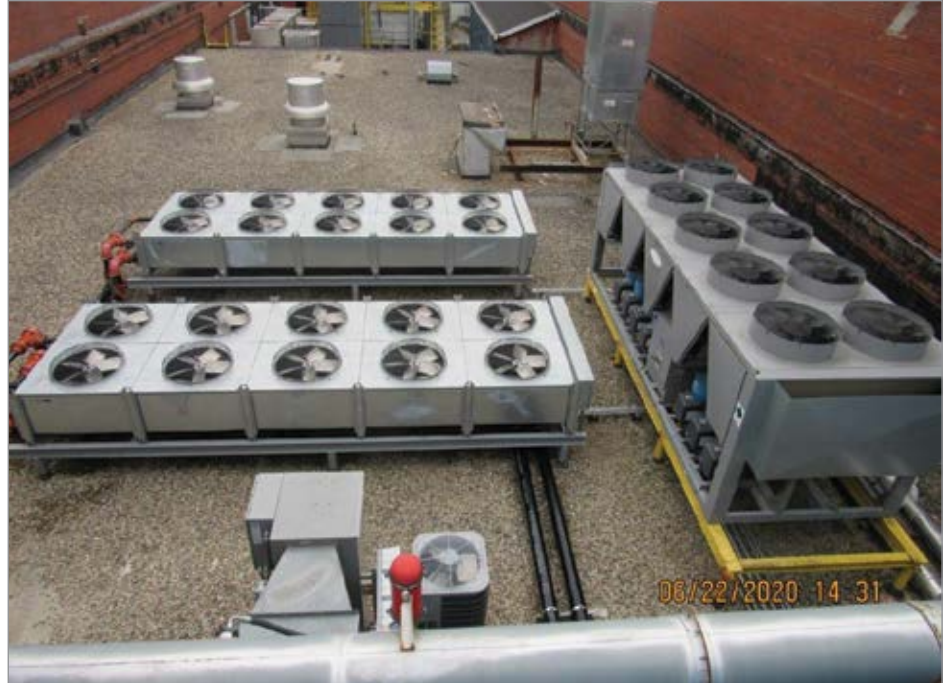
The free-cooling winter cooler installed at the Marysville, Michigan plant.
