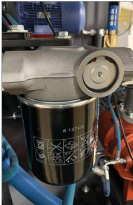
The thermostatic bypass valve on this unit is built into the oil filter housing. Photo courtesy of Ozen Air Technology.
