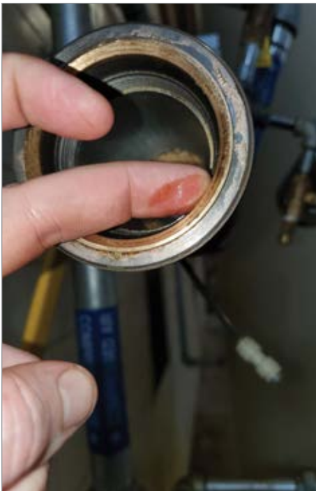
Oil in the compressed air piping downstream of the dryer pointed to the potential problem with the desiccant dryer's inability to maintain the proper PDP.
