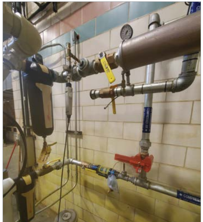
Shown is the test setup used to help validate the cause of the dryer problem.
