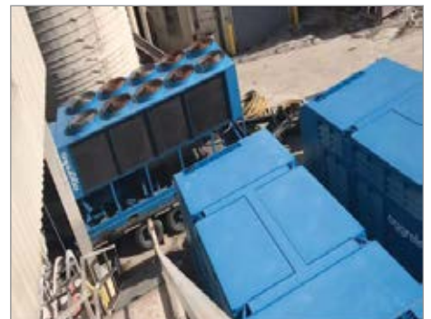
Cool air delivered by the unique compressed air system gives the glassware manufacturer the ability to extend furnace maintenance from one year to two years, significantly increasing plant uptime.
