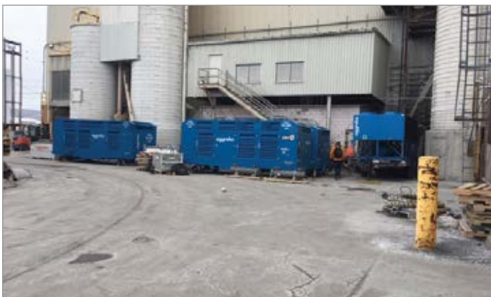
A large manufacturer of consumer glassware products has been able to save $9 million monthly in operational costs by extending the maintenance intervals of its refractory furnace, thanks to a compressed air system featuring an oil-free air compressor, heat exchanger and chiller.
