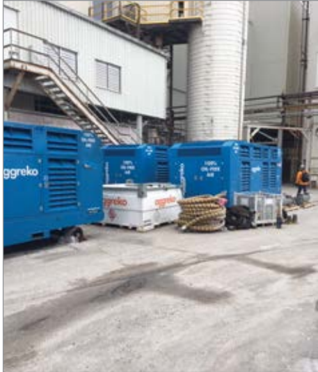
The compressed air system at the glassware products facility uses a heat exchanger in combination with a chiller to deliver compressed air to the company's refractory furnace at a temperature of 45°F (7.2°C).
