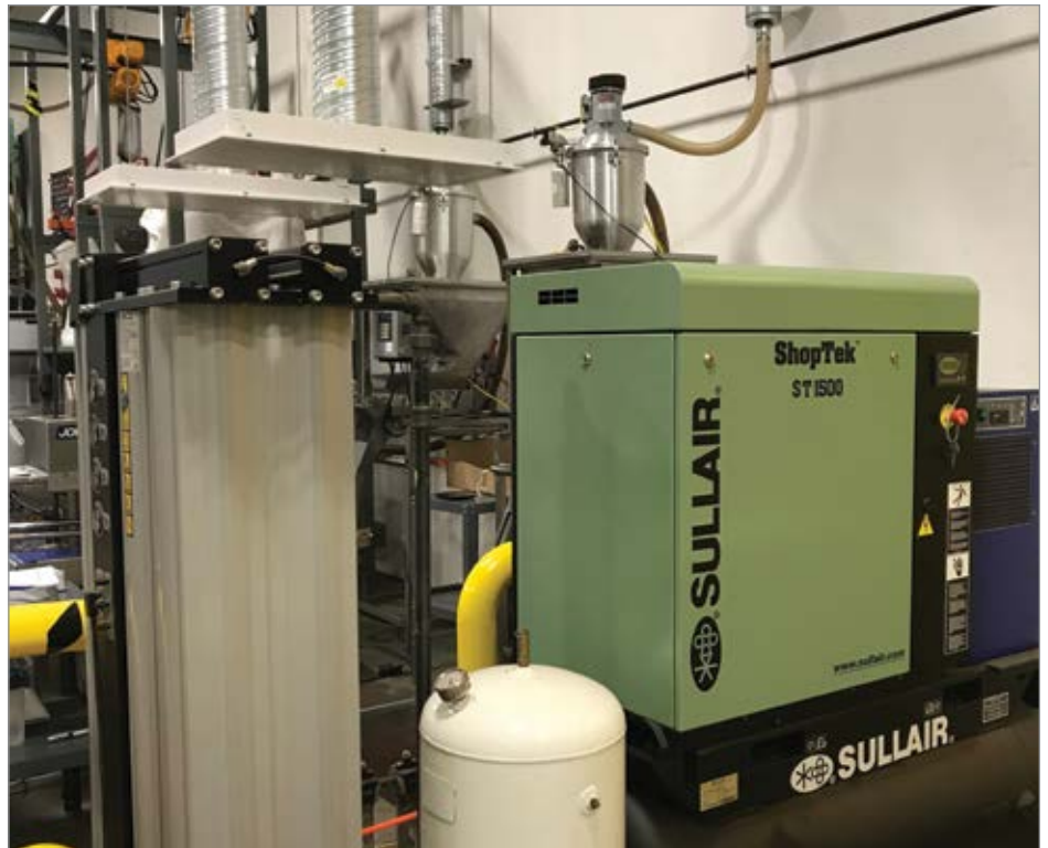
The nitrogen generation system at Death Wish Coffee includes a Sullair ST1509RD, 20-horsepower (hp) rotary screw air compressor and a nano GEN2-2130-Plus nitrogen generator system.
