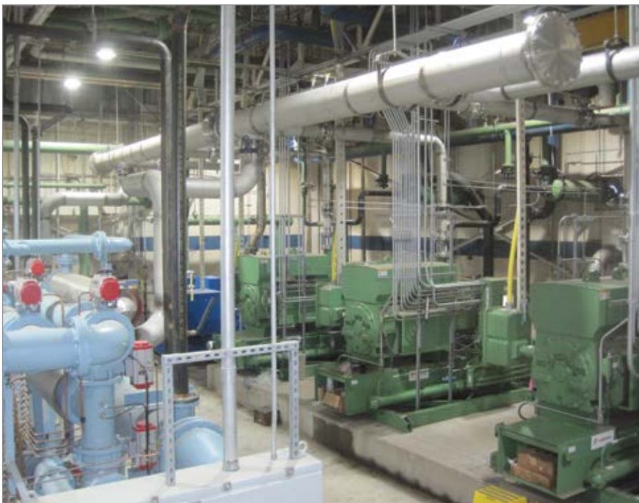
The upgraded compressed air system at KTP has reduced energy consumption by approximately 9.2 GWh. (Photo courtesy of Universal Compressed Air.)
