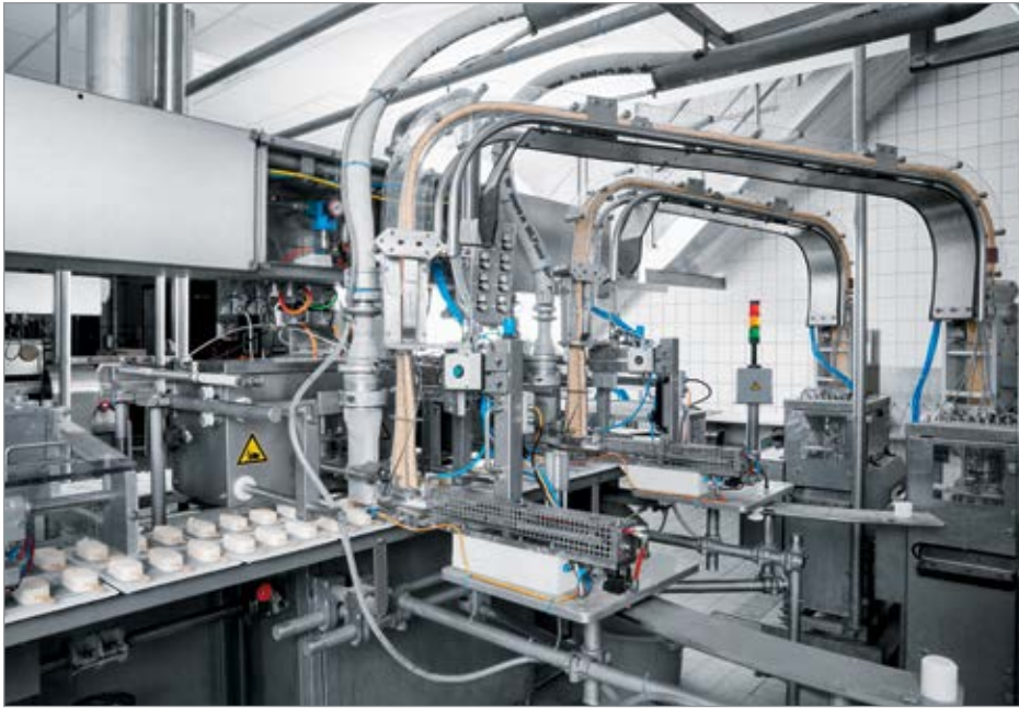
With an energy efficiency module, the Unilever ice cream plant gains visibility into compressed air powering pneumatics on its ice cream production lines, in turn, helping to reduce compressed air consumption.
