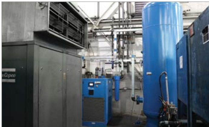
The decision to store air receiver tanks inside, or outside of a facility are driven by multiple factors, including space considerations and the local climate.
