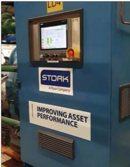
The compressed air system's master controller is used to optimize the performance of the plant's low- and high-pressure compressed air systems.
