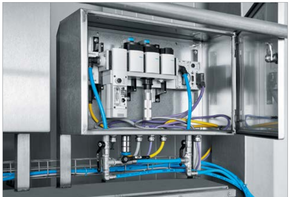
Housed in a cabinet, the Festo energy efficiency module automatically monitors and regulates compressed air powering pneumatics used at the Unilever plant to produce the Magnum brand of ice cream bars.
