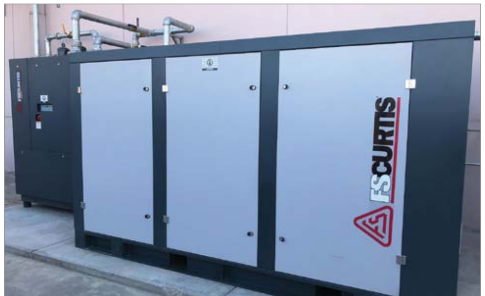
Rotary screw air compressors often provide plants with the biggest opportunity for improvement and savings.
