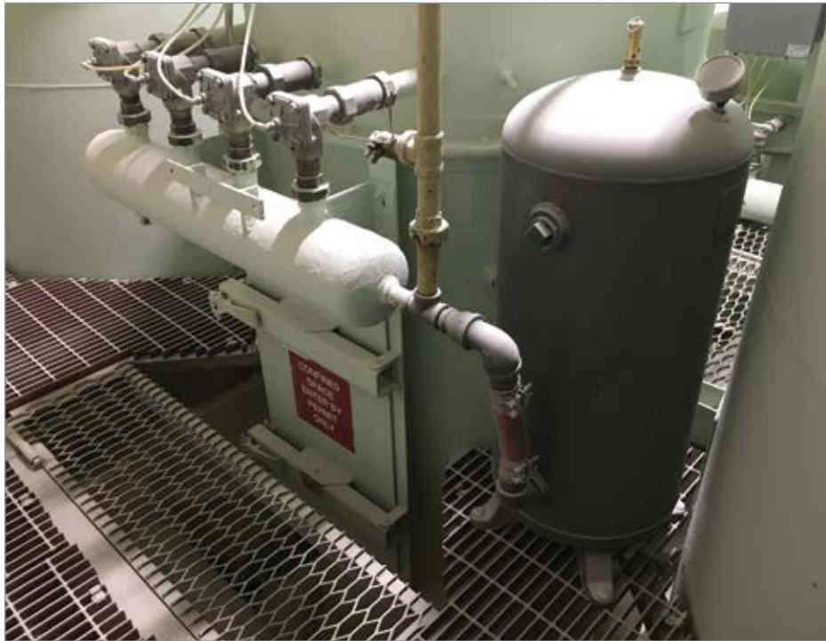
Figure 2: A 60-gallon receiver was added to each problematic dust collector to provide more available compressed air volume per cleaning pulse. The extra storage provided a noticeable increase in pulse strength, popping the bags better for cleaning.
