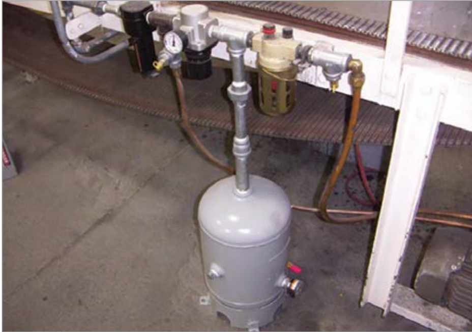
Figure 4. Shown is single-line convector to storage used for a process press. Air is stored to serve as an emergency control and operates if the main air system is disabled.
