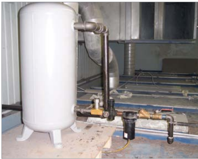
Figure 5: This flow-restricted receiver was installed at the garment plant to solve the problem of transient airflows that were starting a second air compressor.
