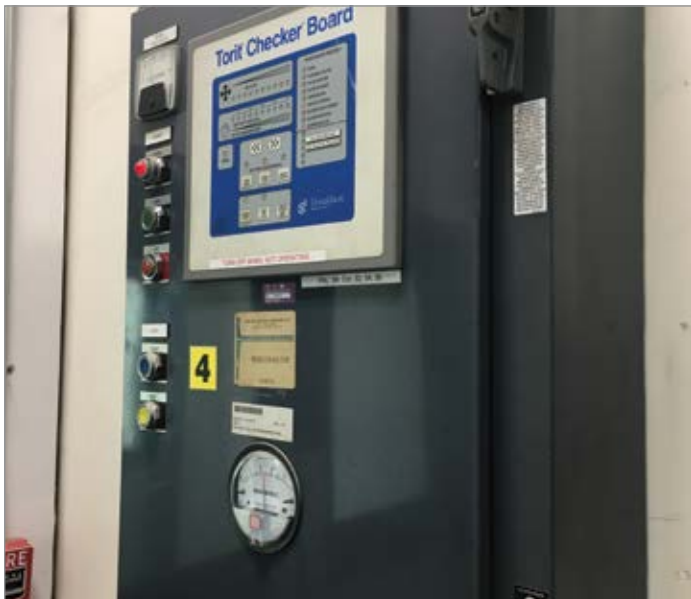
Sophisticated dust collector control panels can make sure the dust collector cleaning system is working correctly and compressed air consumption is held to a minimum.
