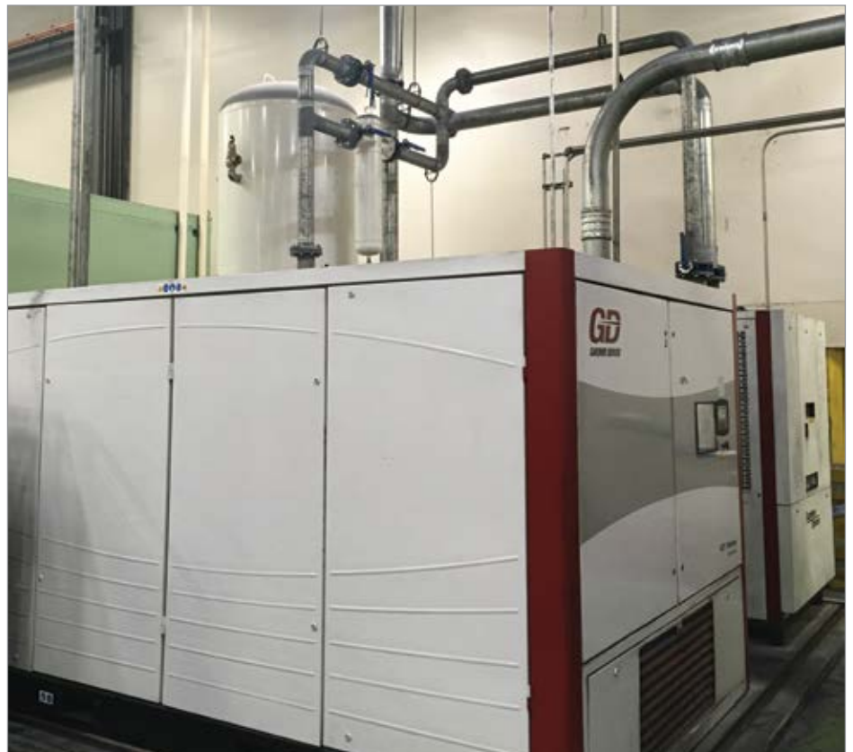
Shown is the 300-hp VSD air compressor installed at SumiRiko's Midway facility to help hold down costs of compressed air delivered to production areas.
