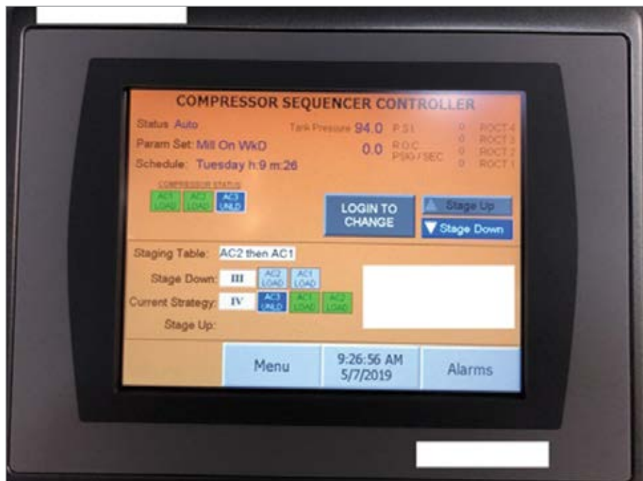
Figure 1: A typical PLC-based control system screen.
