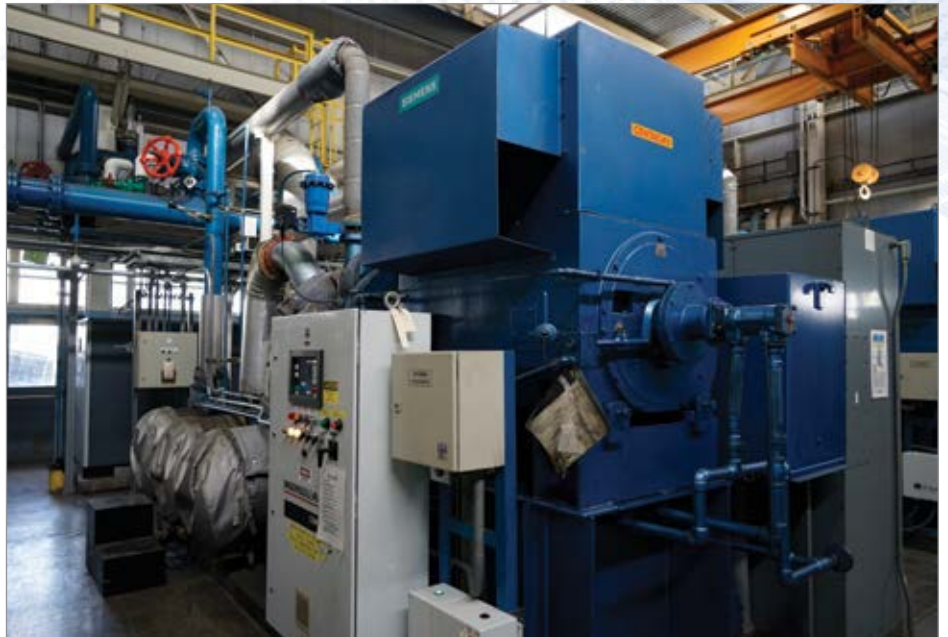
A total of seven Ingersoll Rand centrifugal air compressors are used to power production at a automotive plant spanning 115 acres.
