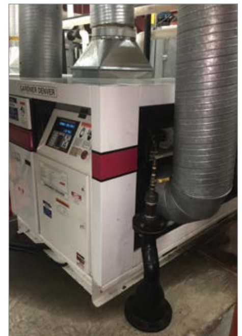
Installed in a hot boiler room, this modulating rotary screw air compressor consumed excessive power and required air conditioning to keep it running.
