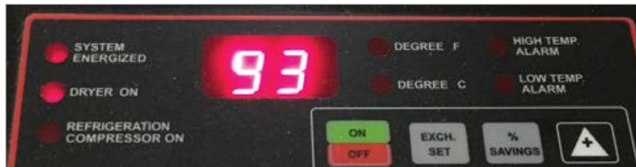
The display panel of the cycling air dryer reports an average energy savings of 93%.
