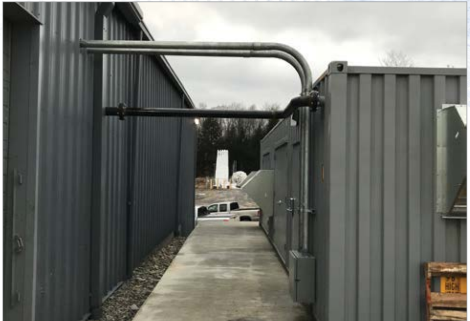
The 40-by-8-foot sea container at GKN houses a complete compressed air system. The unit is located six feet away from the exterior wall of the manufacturing facility.
