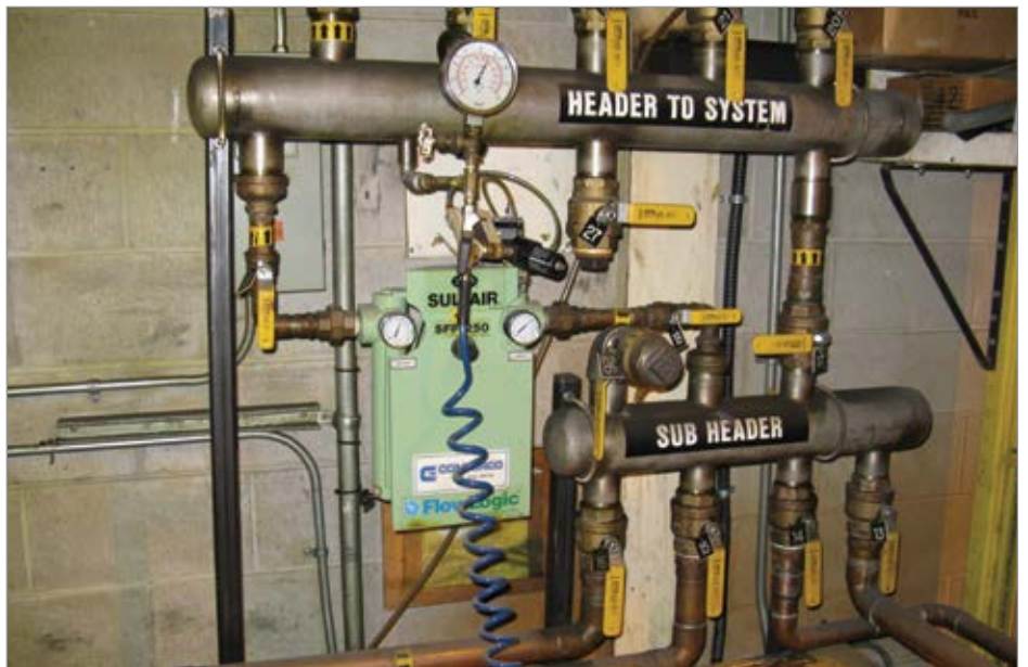
A pressure/flow controller kept plant pressure at a low level and reduced artificial demand.
