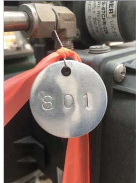
A metal tag with a stamped number identifies the source of a compressed air leak.
