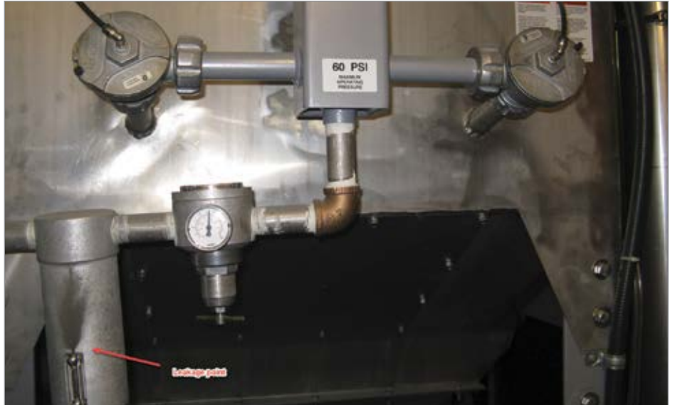
A poorly adjusted blast valve and leakage created problems with this dust collector.
