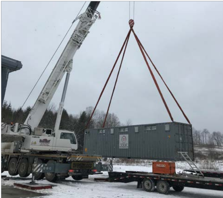
A crane deftly places the sea container into place at GKN. The container houses the entire compressed air system used to meet the air demands of the manufacturing facility.
