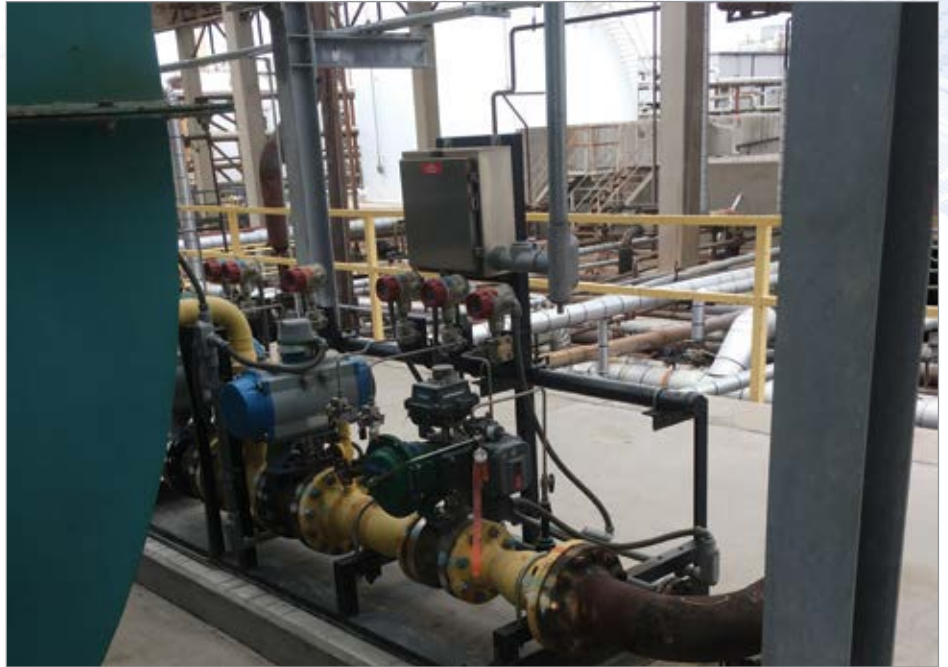
A compressed air leak detection survey can take as many 12 weeks to complete. Engineering tape wrapped around leaks, such as the one shown here, makes them easy to spot for repair.
