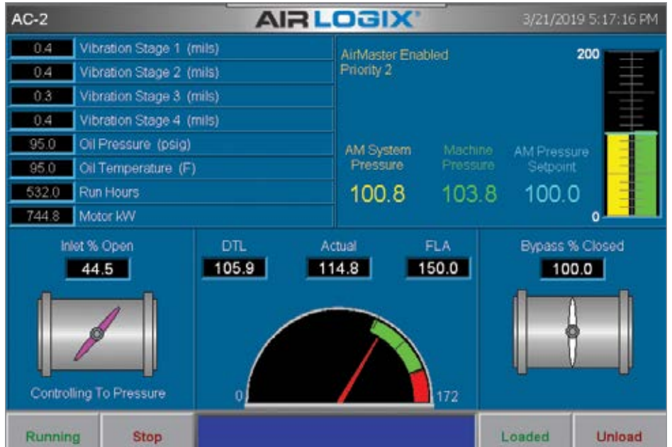
The main screen of an AirLogix local controller shows the DTL minimum limit, which is automatically calculated and adjusted based on air density entering the air compressor and its discharge pressure. The green area in the meter indicates the throttle range for a machine in operation based on these conditions. It also displays critical variables, such as vibration and system pressures.
