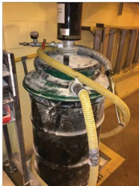
The distillery uses compressed air powered drum vacuums for cleanup, which is an inappropriate use of compressed air and not uncommon at many plants.
