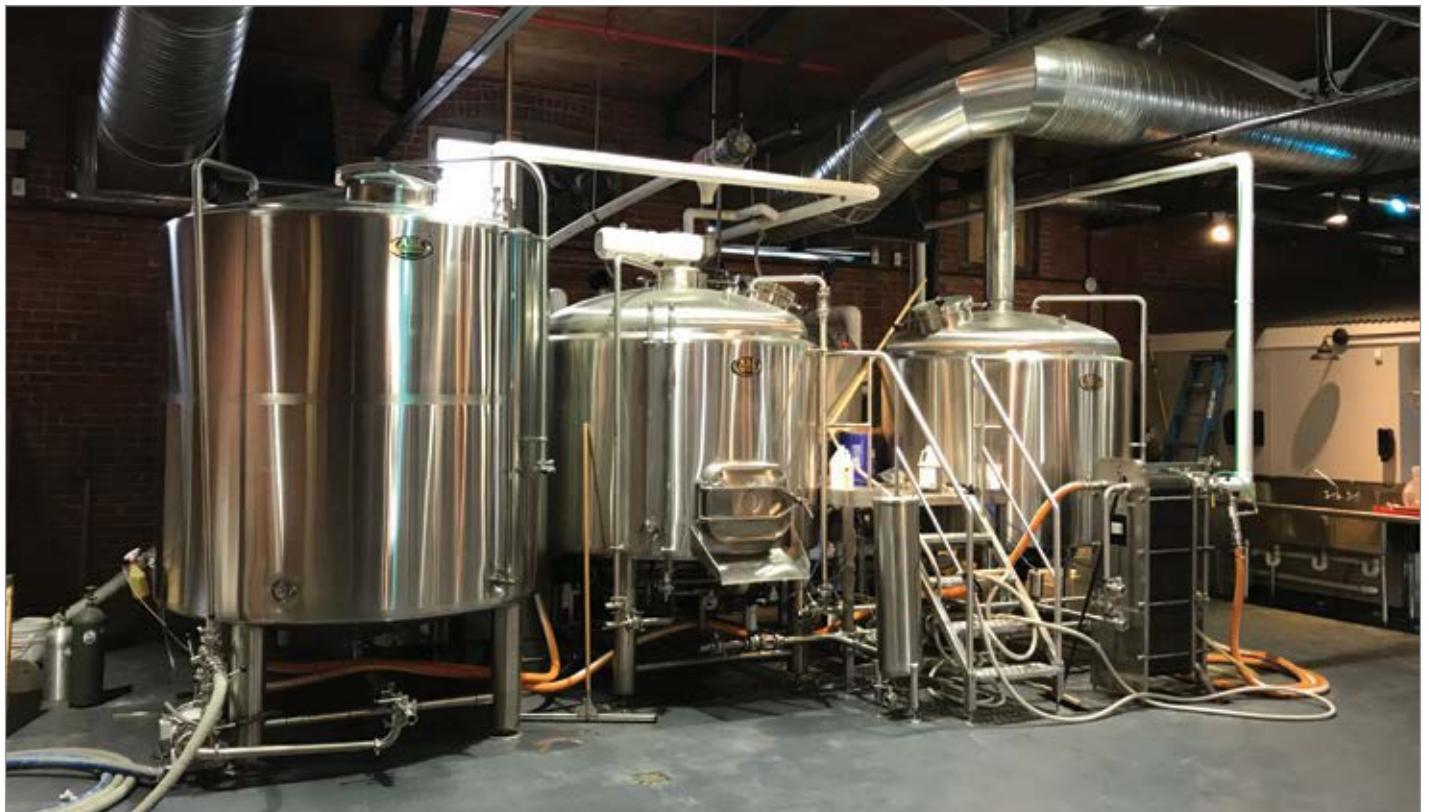
A steady and reliable flow of compressed air is crucial to the brewing process at Five Churches' 20-barrel (bbl) brewhouse.
