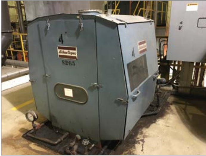
Figure 1: An air compressor has performed reliably for decades, but the aging unit needed to be replaced with a more modern, higher efficiency air compressor.
