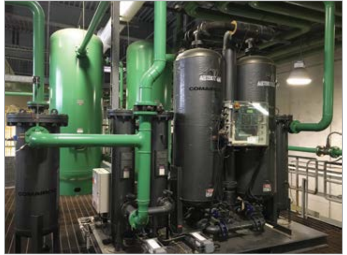
This dryer regenerates infrequently due to lower moisture loading and dewpoint control.
