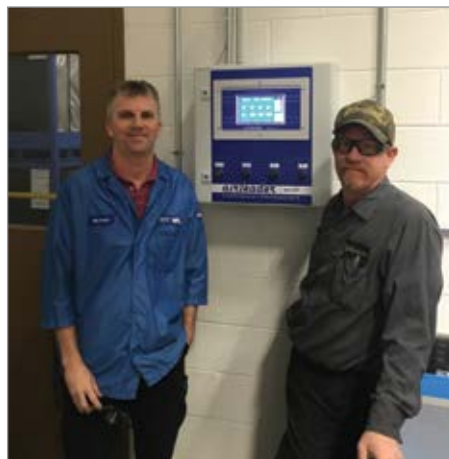
North American Lighting Maintenance Service Manager Michael Westerfield (left) stands next to the Airleader Master Controller with Sean Wisner of Brabazon Pump, Compressor and Vacuum.
