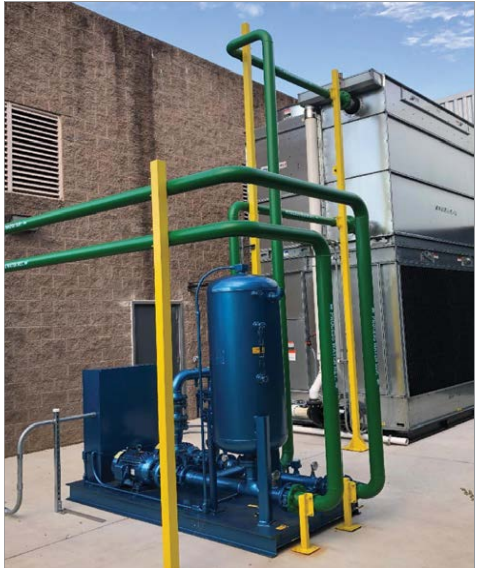
The cooling tower and pump skid at the 1888 Mills facility.
