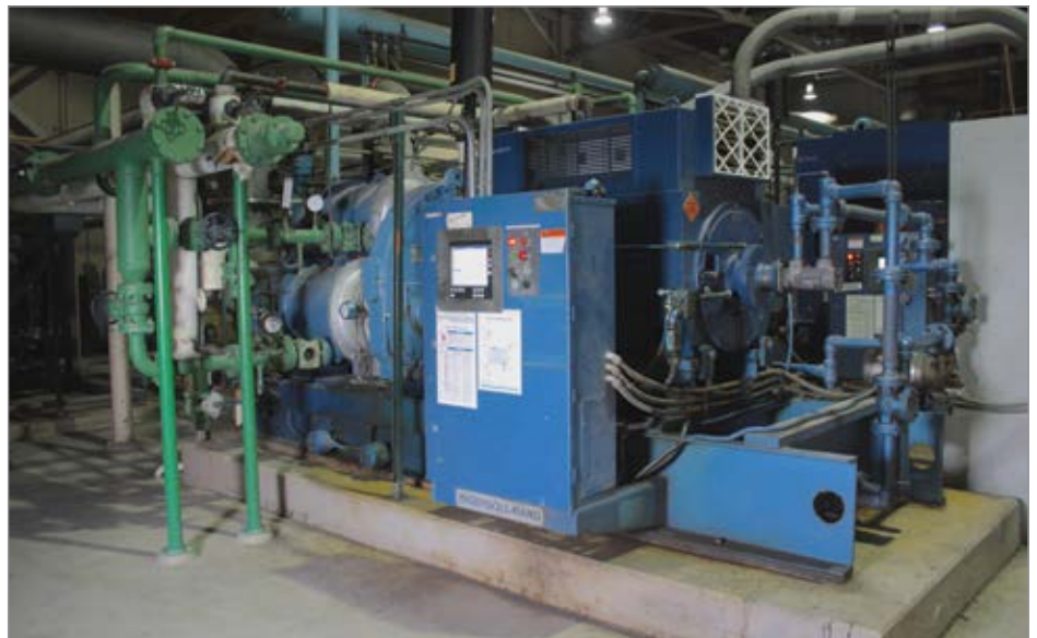
An Ingersoll Rand centrifugal air compressor equipped with a Bay Controls Control System at one of the manufacturer's 10 plants.
