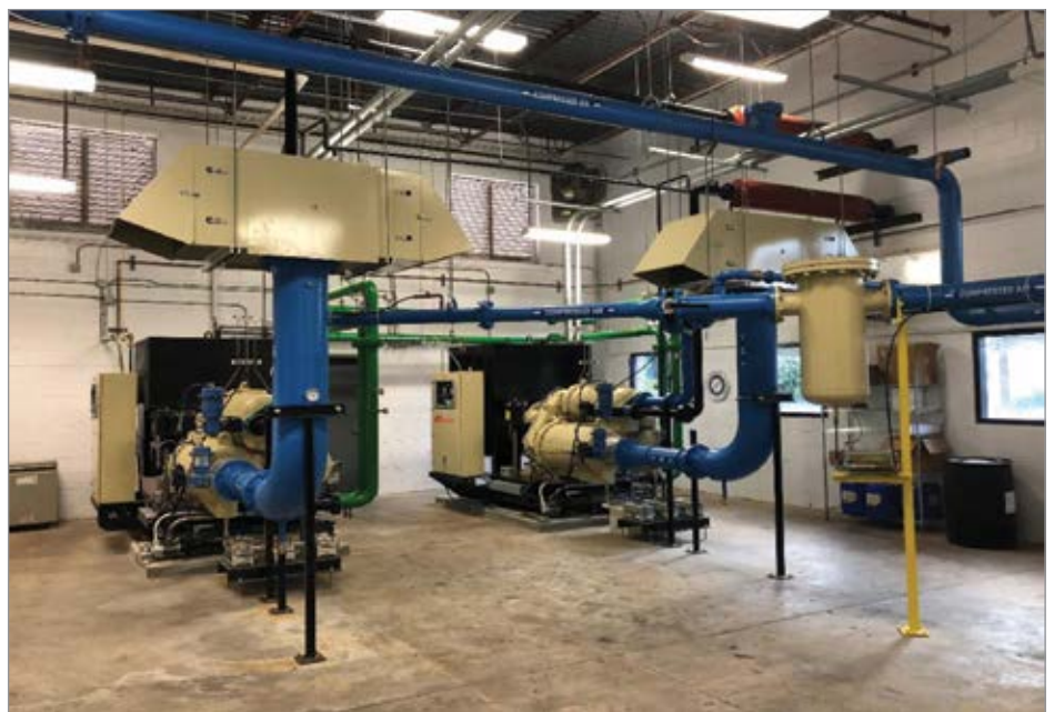
1888 Mills' air compressor room equipped with two Ingersoll Rand C700 Series 600-horsepower Centac centrifugal air compressors.
