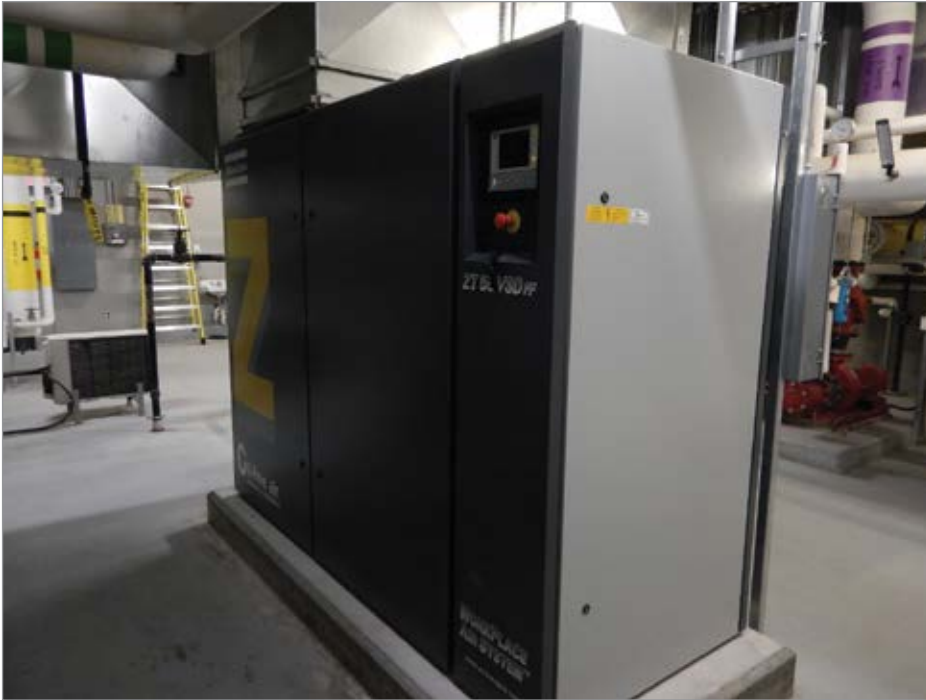
Figure 5: A compressed air dryer is installed internal to the air compressor package, saving floor space.
