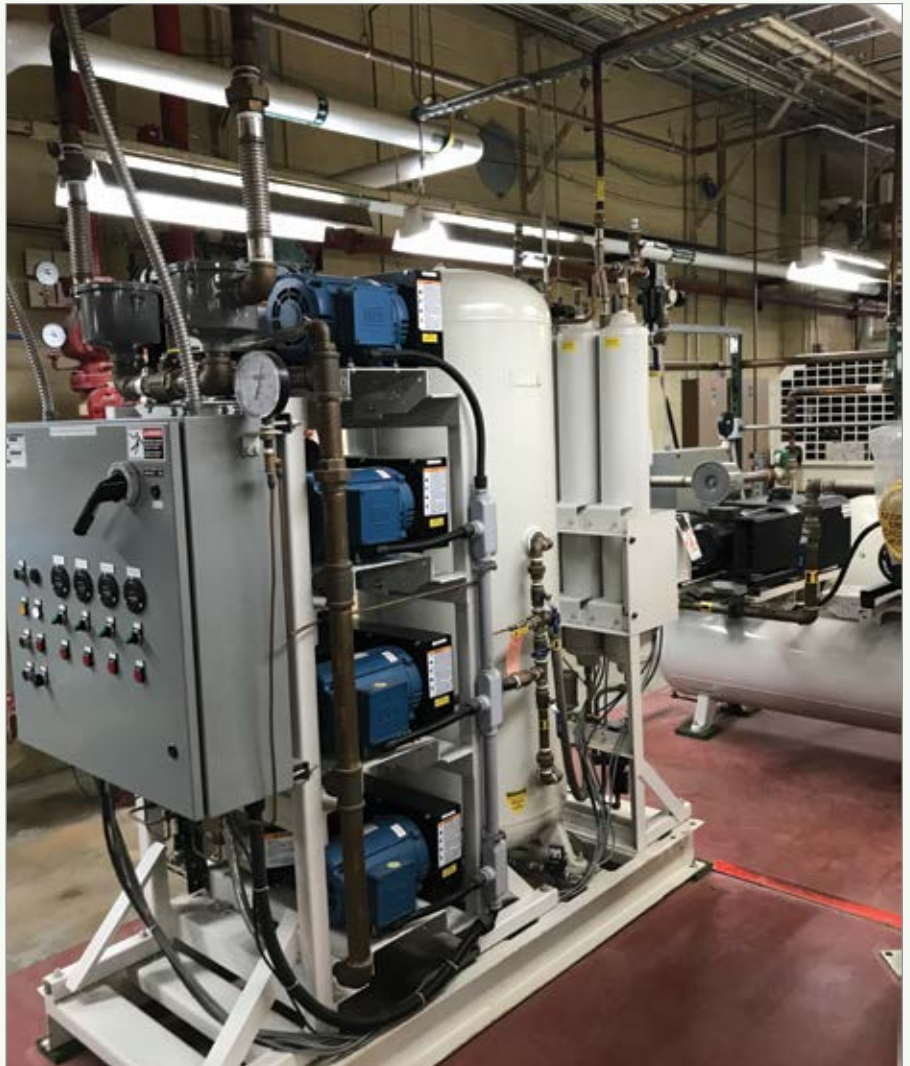
A medical air compressor at a healthcare facility.
