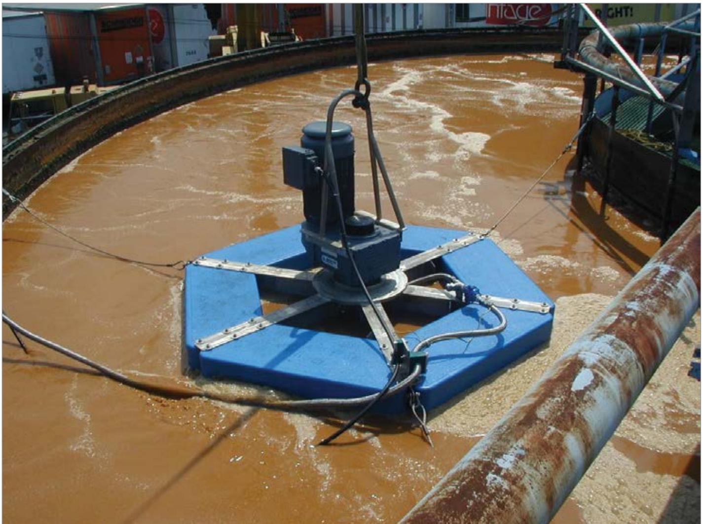
An oxygen system is installed to supplement wastewater treatment processes.
