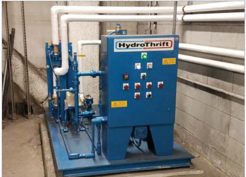
The HydroThrift Heat Recovery System at the Mass Transit Authority Building in Maspeth, NY.
