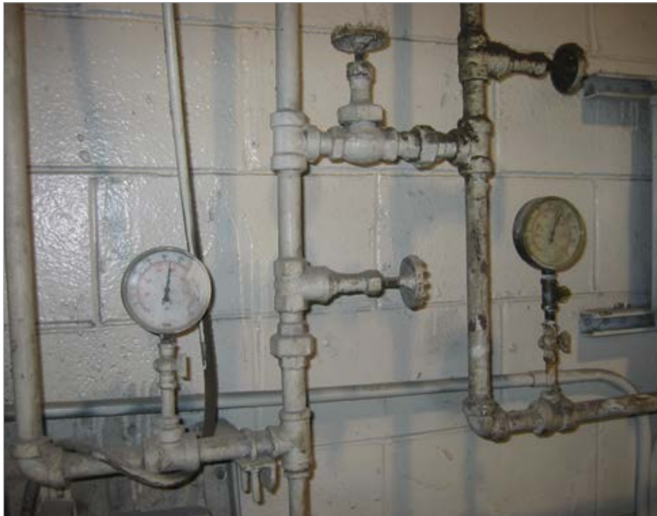
Two pressure gauges were off by 10 and 20 psi respectively.
