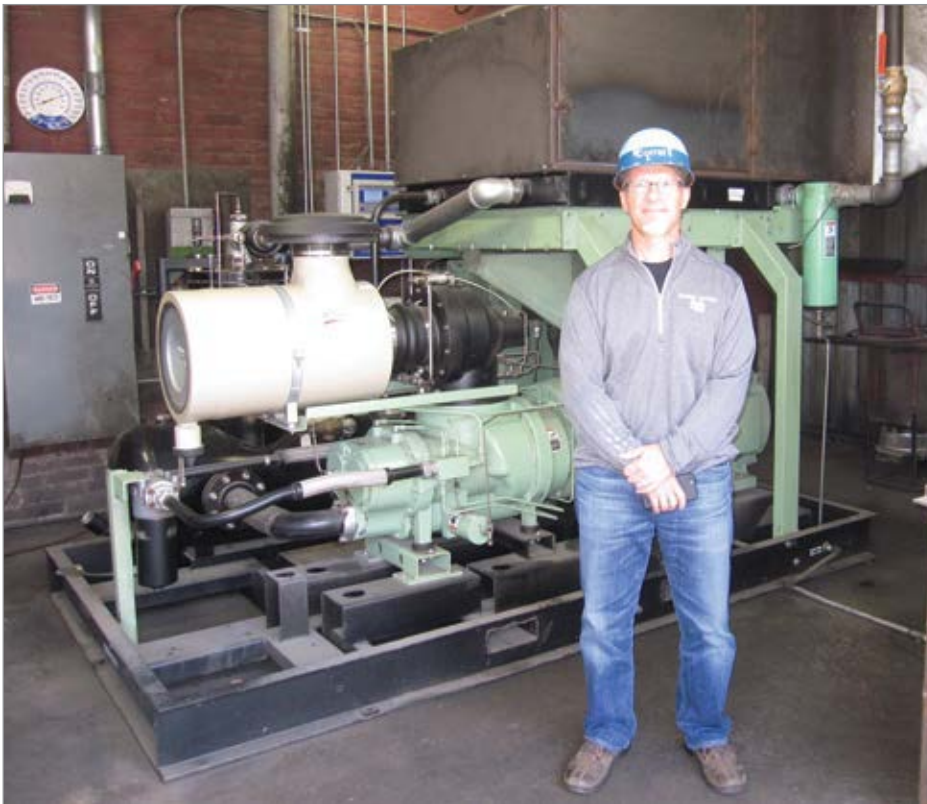
Chicago Heights Steel President Bradley Corral with a new rotary screw air compressor.
