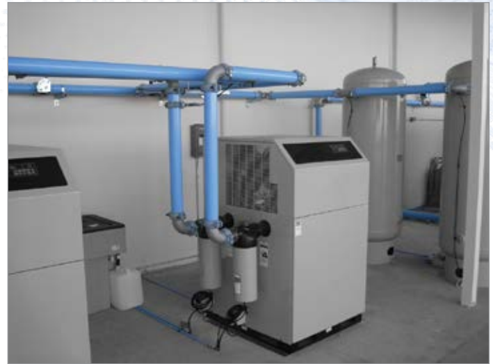
Inlet and outlet aluminum piping delivering compressed air to a refrigerated compressed air dryer and then to storage tanks.
