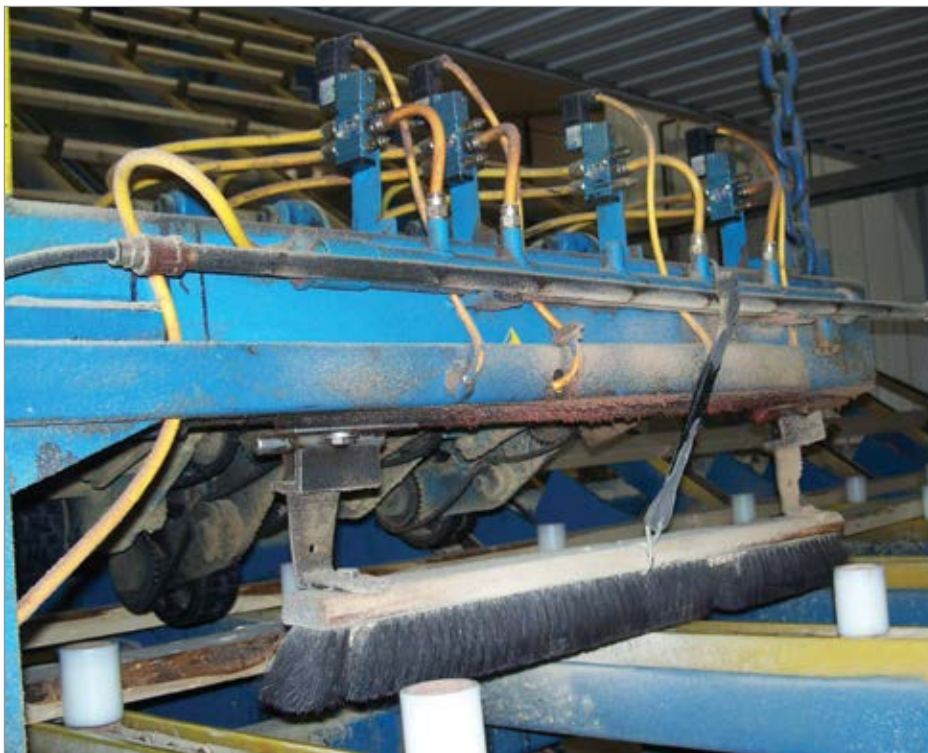
Figure 8: Both compressed air blowing (pipe with holes drilled) and mechanical broom power are used to clear wood chips from lumber pieces. Guess which uses less energy.
