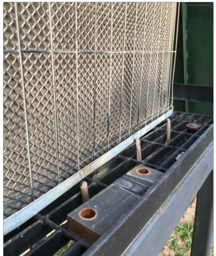
Figure 6: An air conditioning unit was cleaned by a timer controlled blast affecting air compressor control
