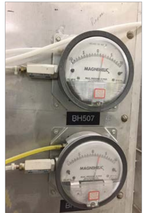
Magnehelic gauge installed with inline filter on clean air port.
