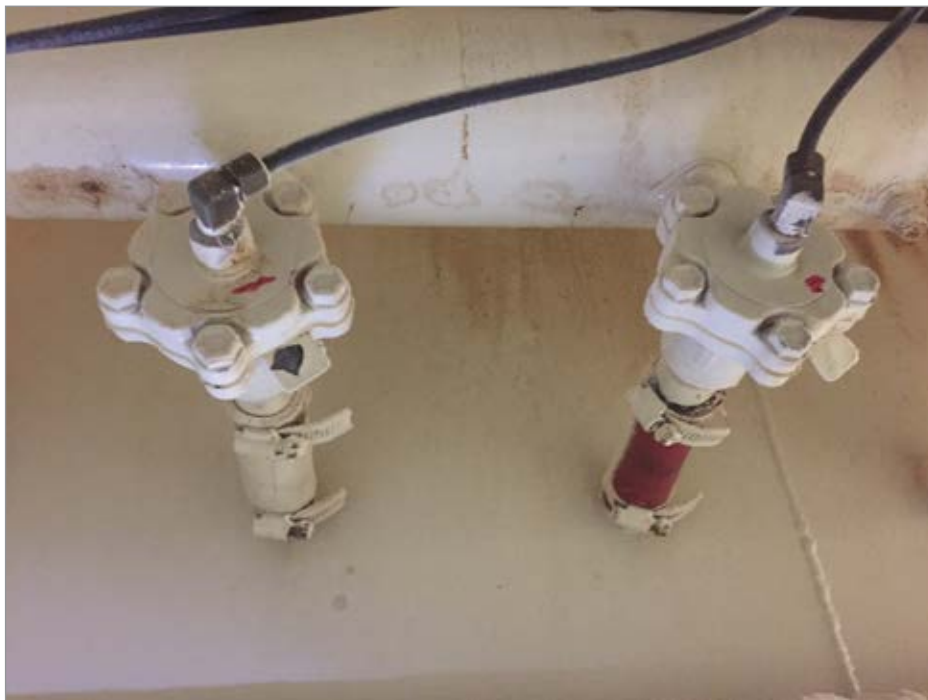
A 20 year-old dust collector with original pulse valve diaphragms. Notice diaphragm tab is painted same color at unit.
