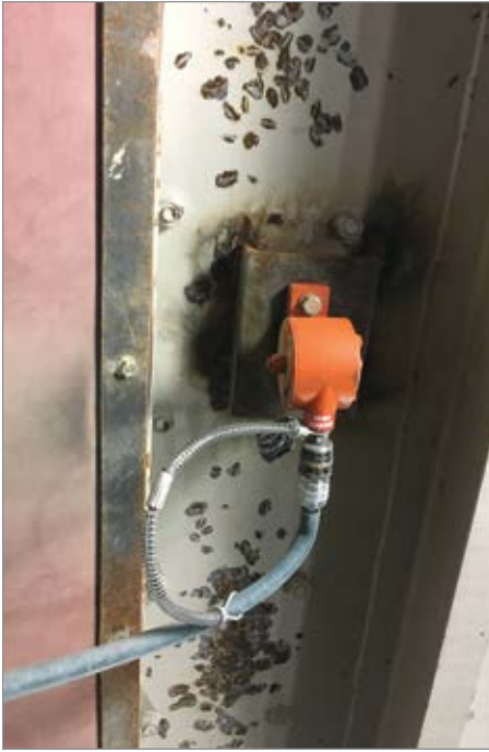
Figure 4: Air vibrators like this could be the reason a second compressor has to run.
