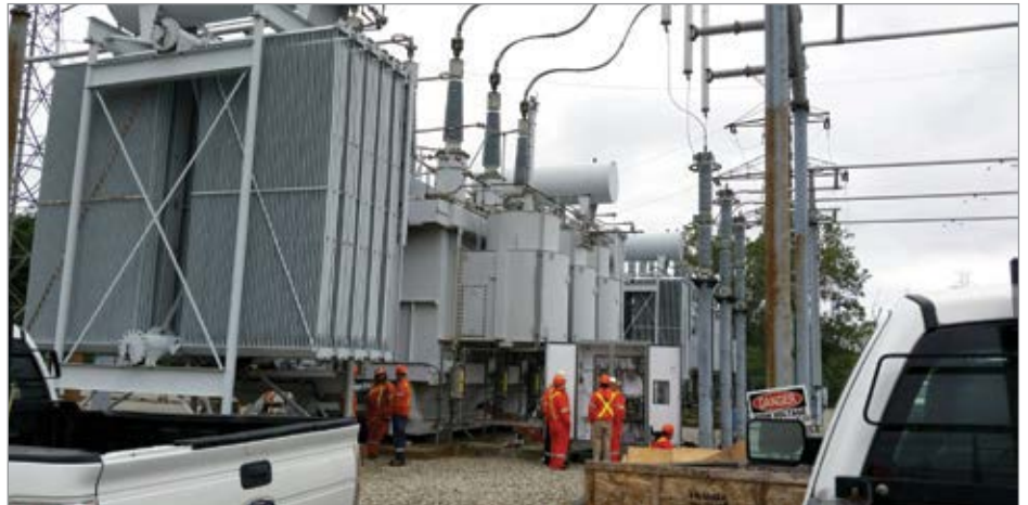
Vaisala partners with DryKeep to enhance the moisture monitoring capabilities of its transformer dry-out system.
