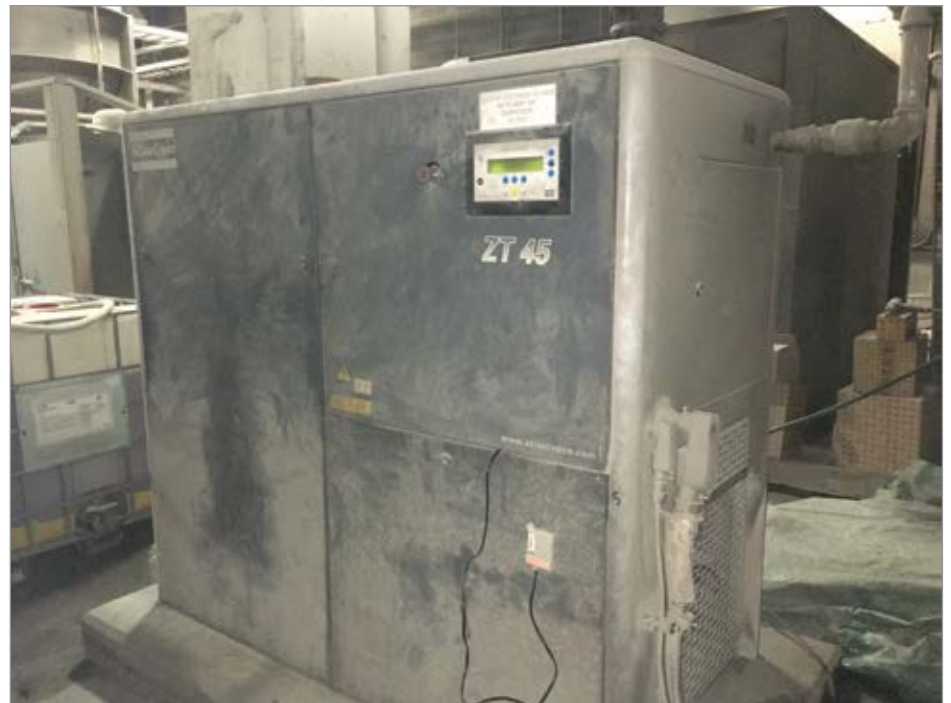
Figure 1: The dusty environment causes maintenance issues at this site.
