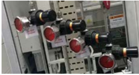
Figure 7. Having two pressure regulators in series causes excess pressure differential and poor pressure regulation.
