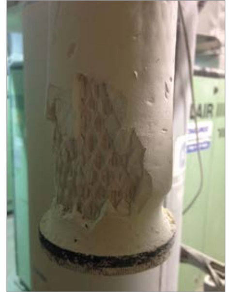
Figure 4: High velocities in the dryer pulverized the desiccant beads clogging the filters, this had been changed a few weeks earlier.
