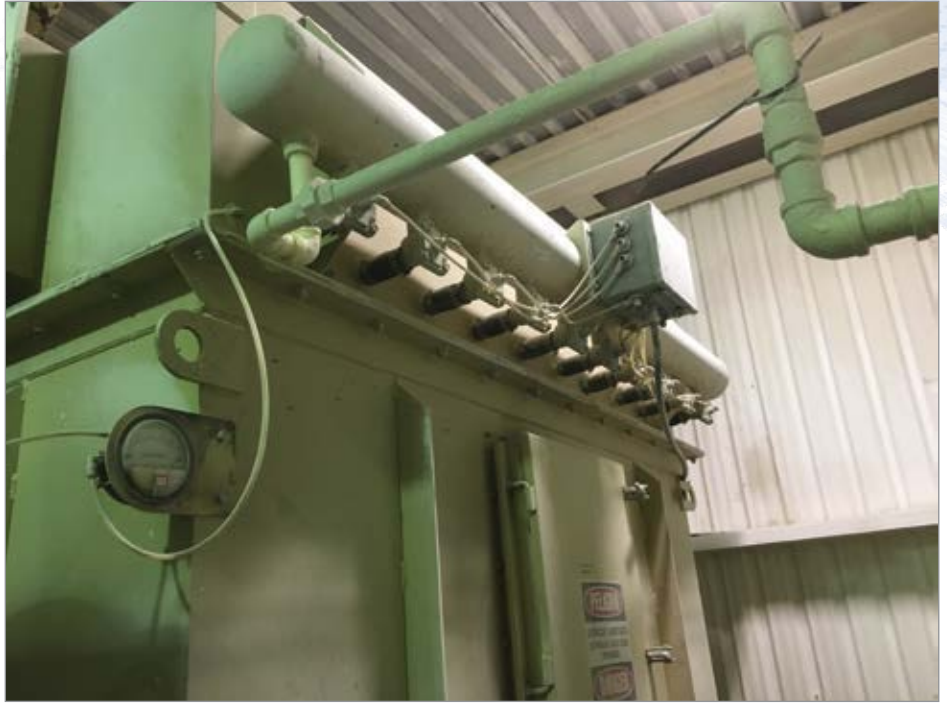
Figure 1: Baghouses represent about 95 percent of the plant compressed air loading
