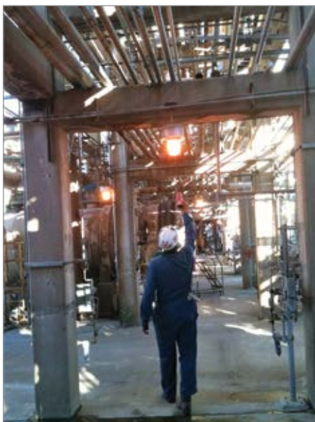
Compressed air leak surveys in the petrochemical industry differ from surveys in "quiet" manufacturing or commercial industries.
