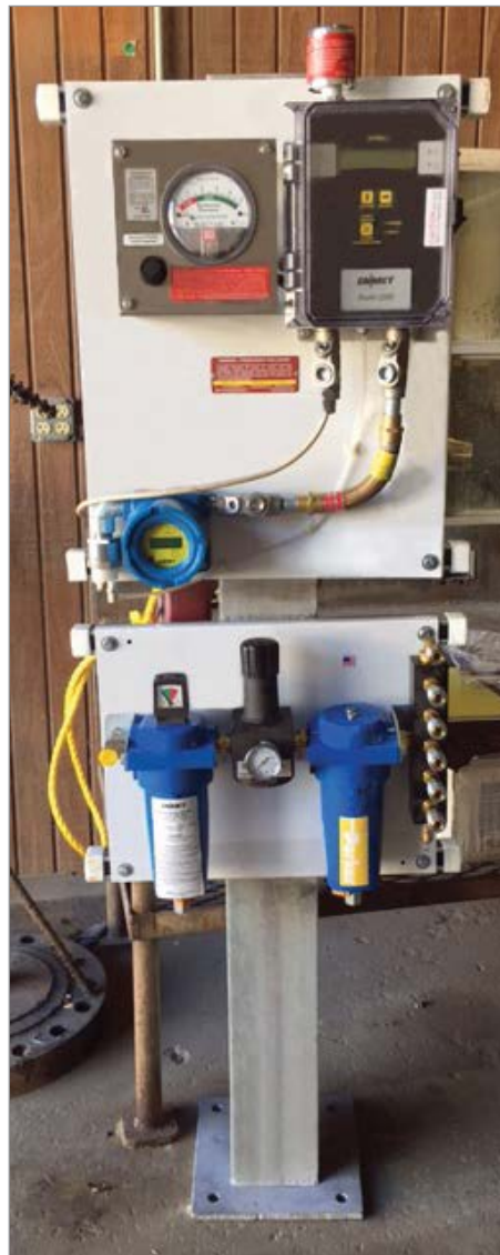
A custom designed AFS-100 air filtration system with a ProAir 2200 carbon monoxide monitor.
