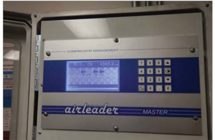
Figure 5: This controller runs the air compressors with best efficiency at full load and varies the flow of the compressors with variable capacity control.
