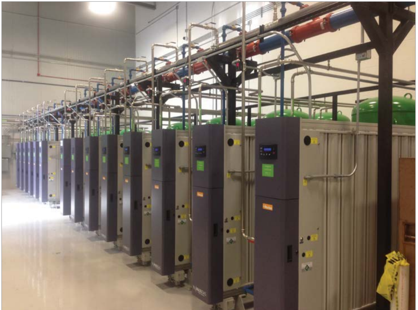
Parker dh Multibank Nitrogen Generators at a Coffee Packager
