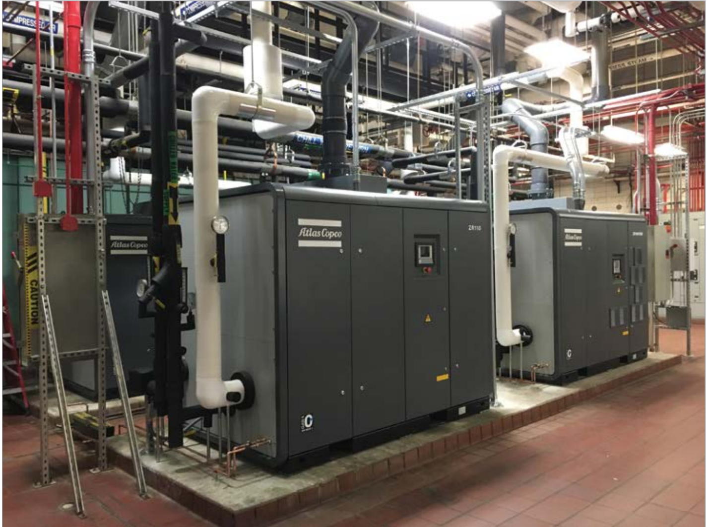
New Air Compressors at NIST
