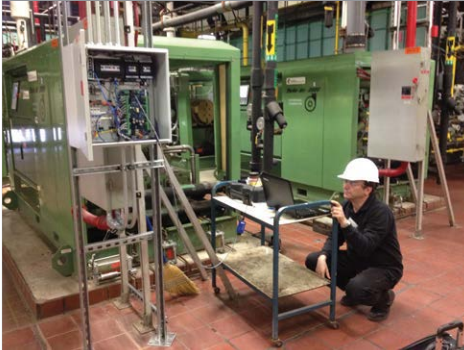
Commissioning of the ReMaster System at NIST
