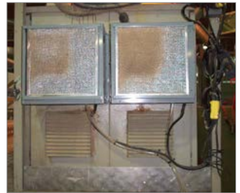
Figure 2: Thermostatically controlled refrigerated coolers were retrofitted to the cabinets and consumed about 96% less energy
