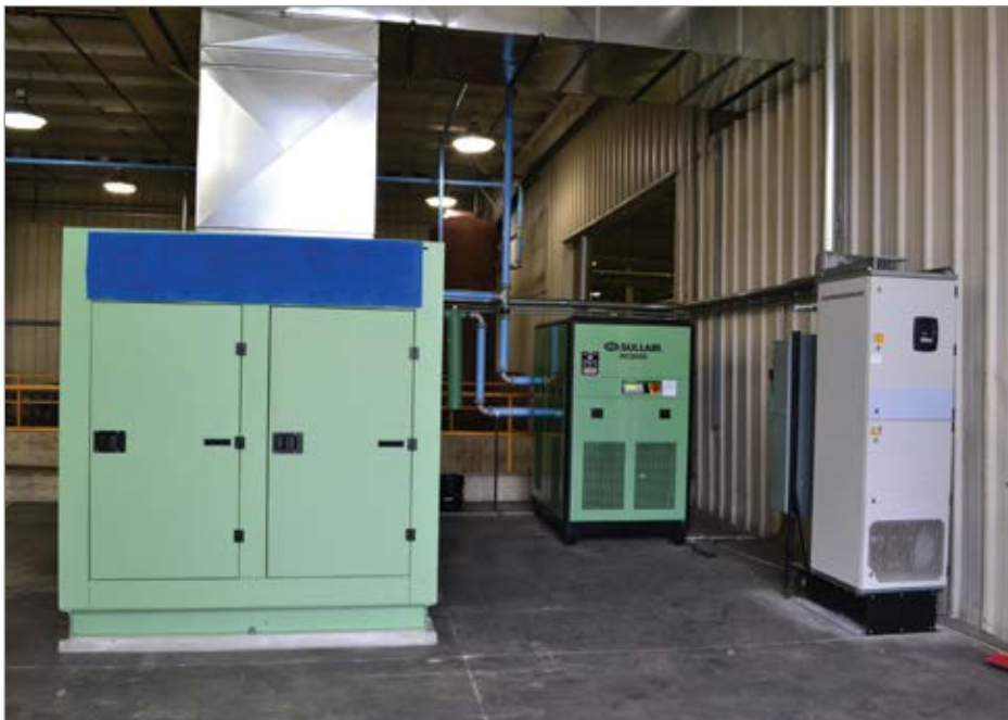
The new compressor room location included the installation of new cooling air exhaust ducting from the air compressor for heat recovery, expanded headers, aluminum distribution piping, refrigerated air dryer, pre- and after-filters, and a new 1550 gallon receiver tank.
