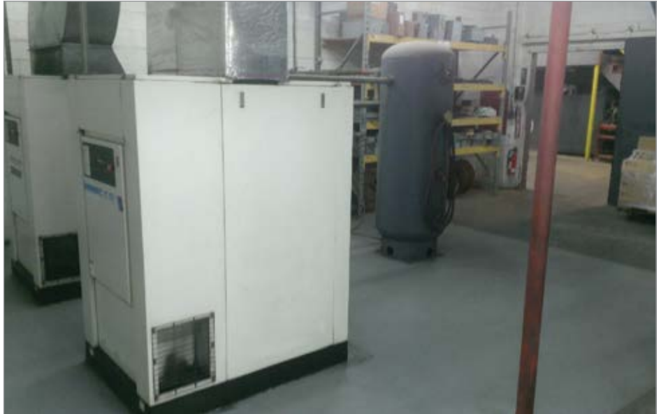
The existing installation had five 50 HP and one 20 HP single-stage, lubricated rotary screw compressors running partially loaded.
