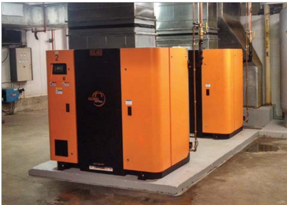
In conjunction with installing appropriate storage capacity, HAECO is also in the process of replacing each pair of 75-hp air compressors with two 50-hp ELGi air compressors.
