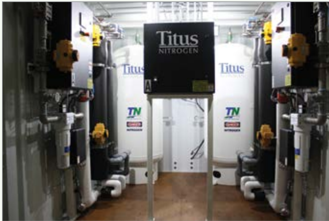
The turnkey nitrogen generation system included PLC-based instrumentation for local and remote control, along with nitrogen storage tanks.
