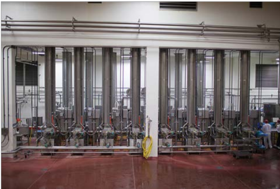
Compressed air leaks are common in the cheese towers at Darigold’s Sunnyside location, so the Energy Team installed flow meters to monitor leak rates.
