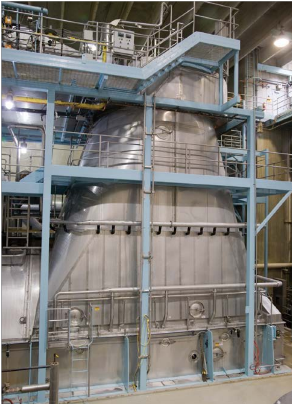
Milk powder dryers are major pieces of equipment within Darigold’s plants.
