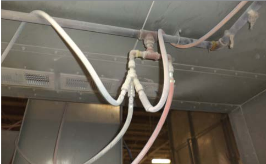
Figure 3: Questionable connection practices caused huge pressure differentials in some areas.
