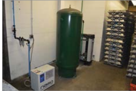
Installed by C.H. Reed, the foundry's nitrogen generation system featured a nano NRC Cycling Refrigerated Air Dryer (left) and a nano N 2 plus Series Nitrogen Generator (right).
