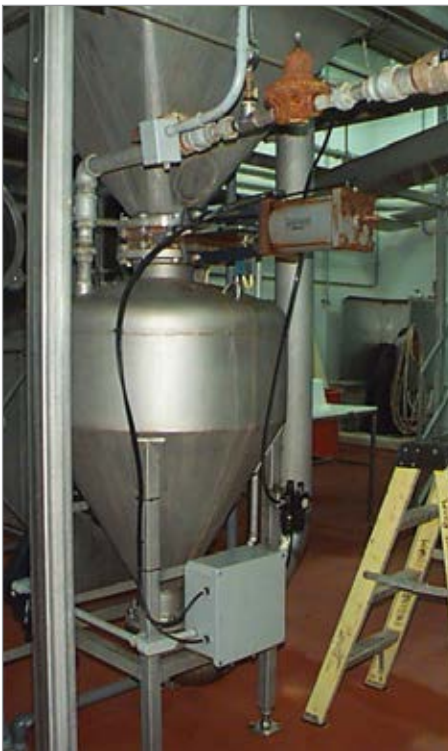
Figure 4: Material is transported pneumatically, causing transient high flow events.
