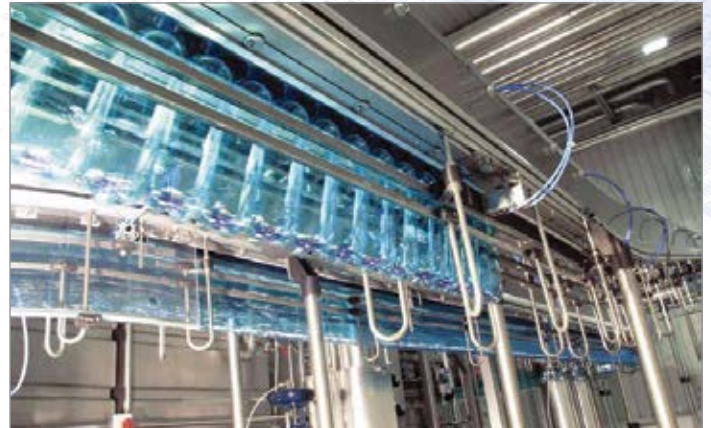
Blow-off applications are common in a great deal of F&B manufacturing facilities.
