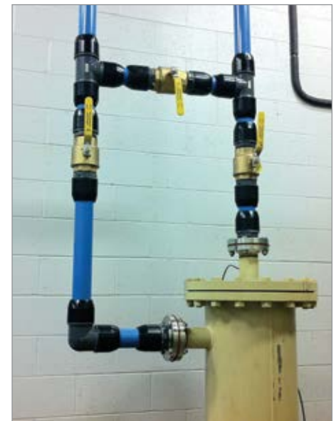
Figure 7: Mist eliminator filter and associated piping
