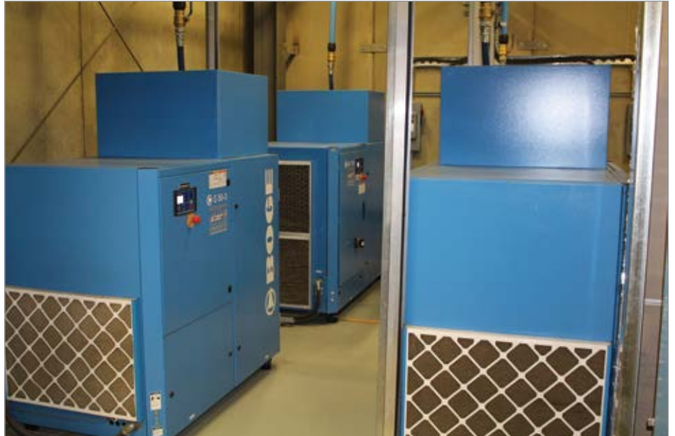
BOGE air compressors installed by Central Air Equipment at Finning International
