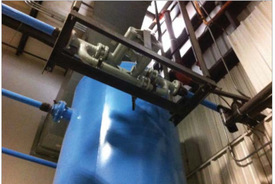
Figure 5: Pressure/flow controller regulating plant pressure to 85 psig (bottom view with tank shown)
