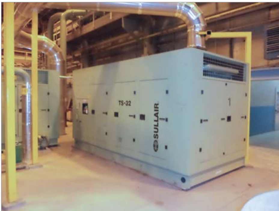
Figure 1: Four large, two-stage, water-cooled compressors with spiral valve control are used as trim capacity.
