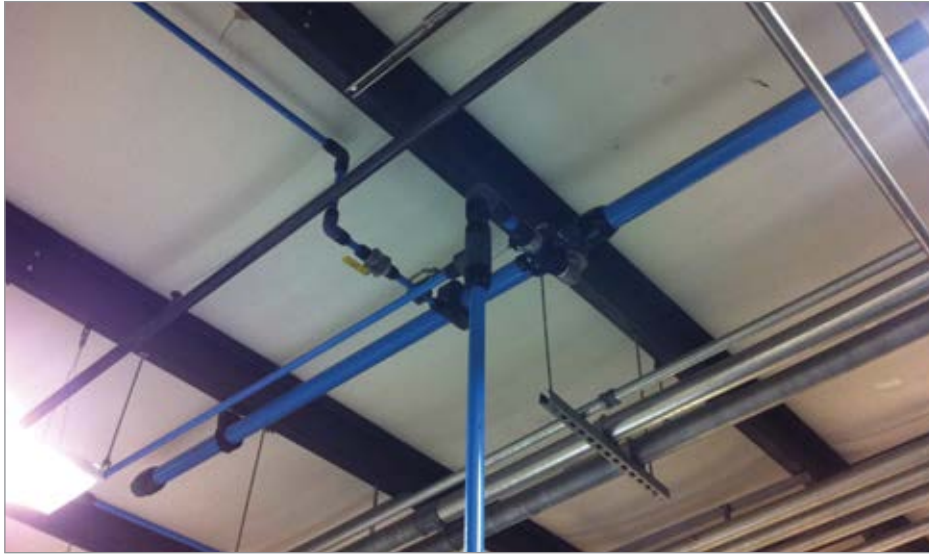
Figure 3: Aluminum piping system — The aluminum pipes are blue in color and slip fit connectors are black.
