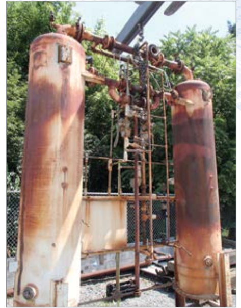
Figure 1: The refinery’s original ORIAD ® Series internally heated reactivated dryer after years of disuse
