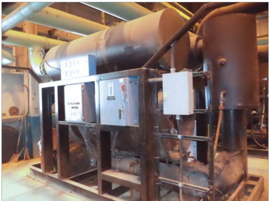
Figure 3: Hybrid-style dryers are used onsite to condition the air for the smelter. This is the 10,000 cfm rated refrigerated part of the combined refrigerated/heated/blower desiccant unit.
