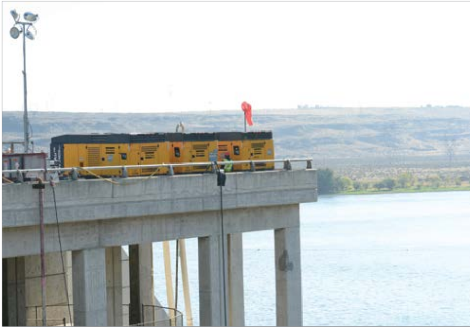
Rental Atlas Copco air compressors at the Wanapum Dam
