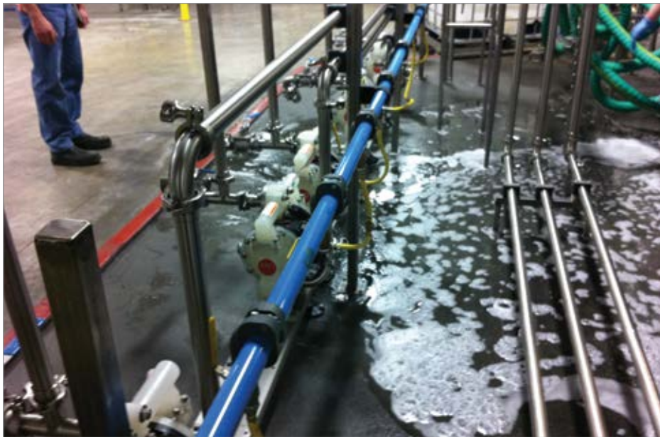
Figure 4: Diaphragm pump header regulated to 55 psig
