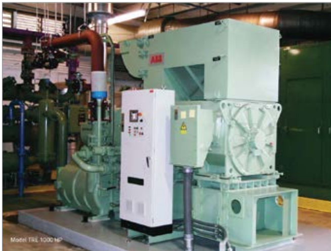
Pictured is a T-series centrifugal compressor from Sullair’s very first installation in Midland, Michigan.
