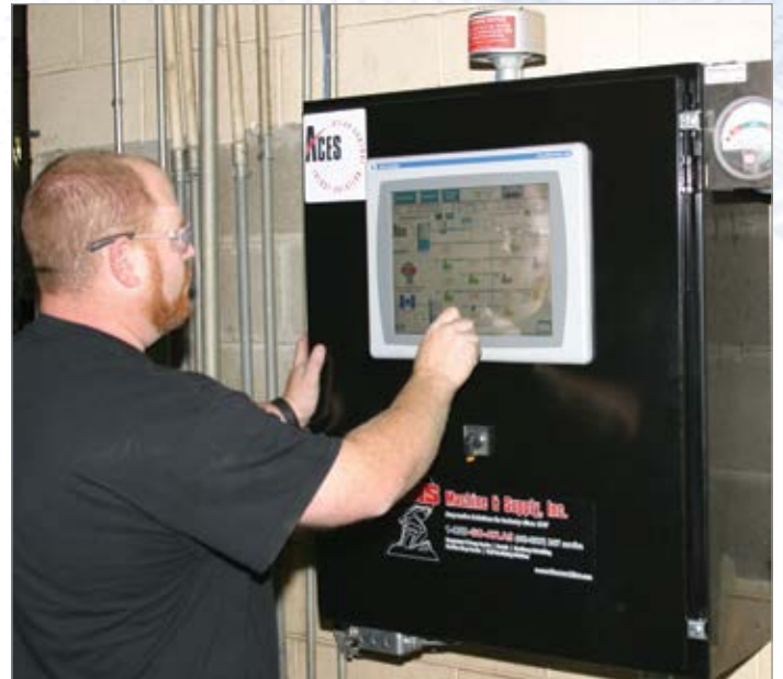
ACES-16 air management system is powerful energy optimization tool.
