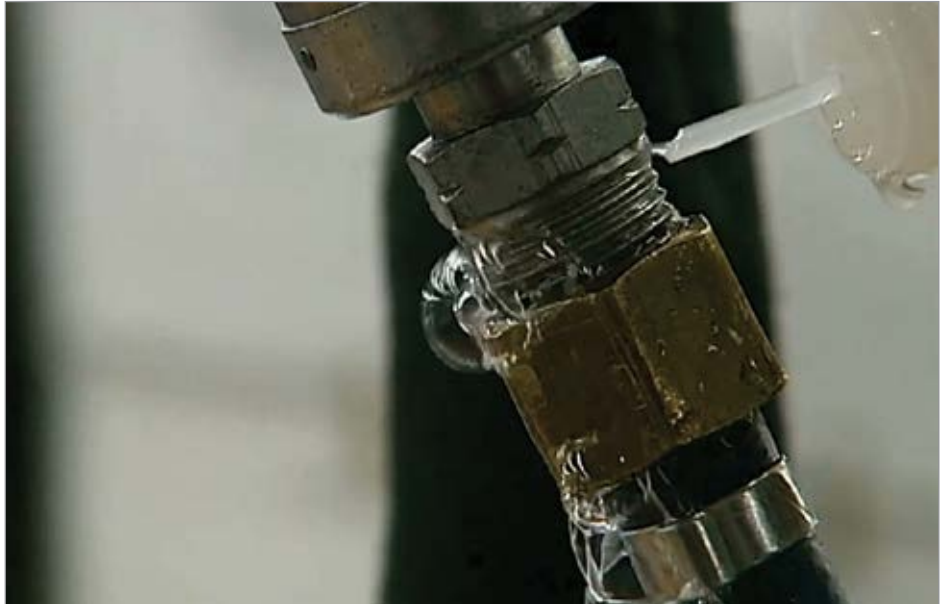
By vigilantly repairing compressed air leaks, Nissan aims to achieve a leak rate of less than 10 percent of compressor output.
