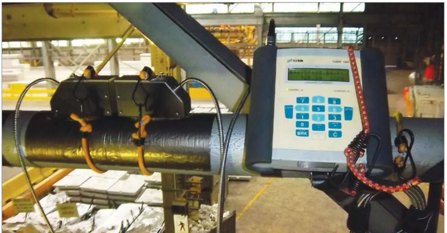
The aluminum plant installed two ultrasonic flow meters — both on the main compressed air headers 60 feet above the floor.
