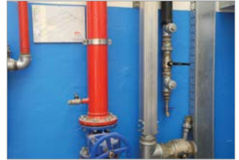
TESEO HBS modular piping for the new compressed air distribution system in the factory of Persico Spa.
