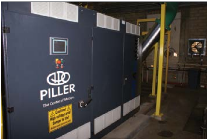
The newest blower was installed in 2013, and provides sophisticated controls.
