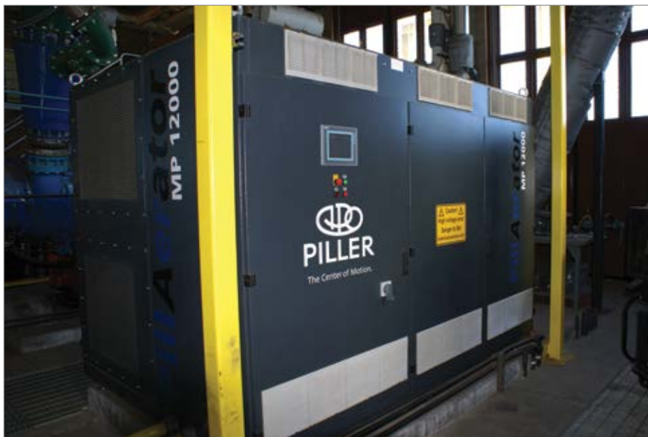
Staff at the Victor Valley Wastewater Reclamation Authority decided to implement new 400-hp blowers to address their aeration needs.
