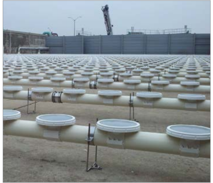
Installing PTFE-coated membranes helped avoid the costly construction of additional facilities.
