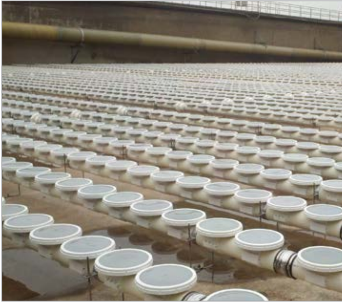
The WWTP of the City of Fort Worth, Texas, installed 70,000 pieces of 9-inch disc diffusers with PTFE membrane coatings.
