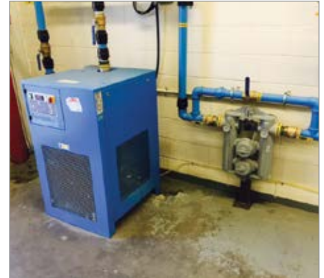
Figure 3: Refrigerated dryer connected to aluminum piping
