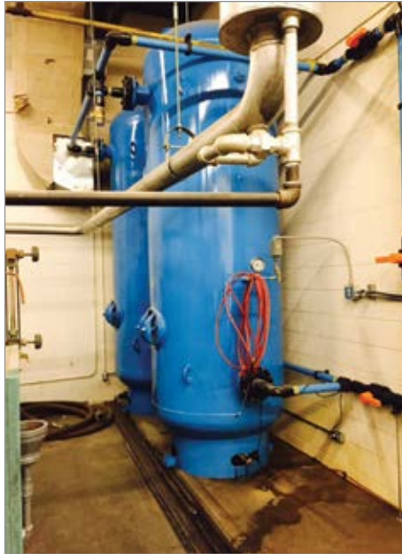
Figure 2: Dual 1060 gallon vertical air receivers with aluminum piping
