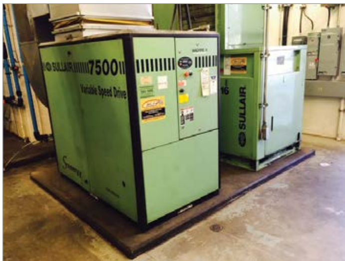
Figure 1: The 100-hp VSD air compressor along with the 75-hp machine
