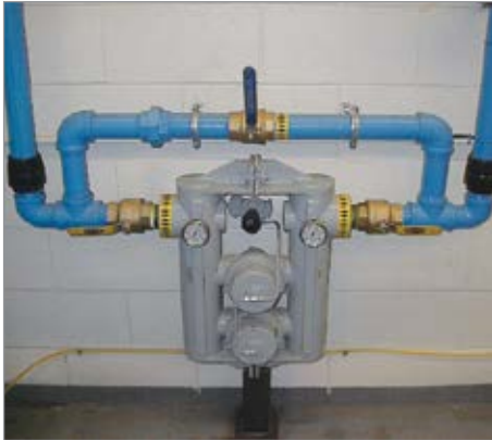
Figure 4: Compressed air flow regulator
