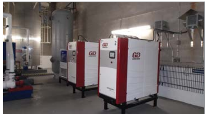
Figure 4: The new air-cooled compressors do not require an external cooler and heat an area of the plant displacing natural gas heat.
