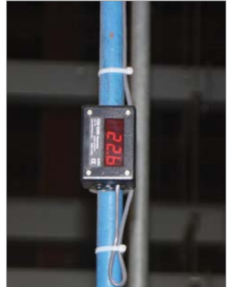
CDI 5200 flow meter serving an individual piece of equipment in a ceramics manufacturing plant
