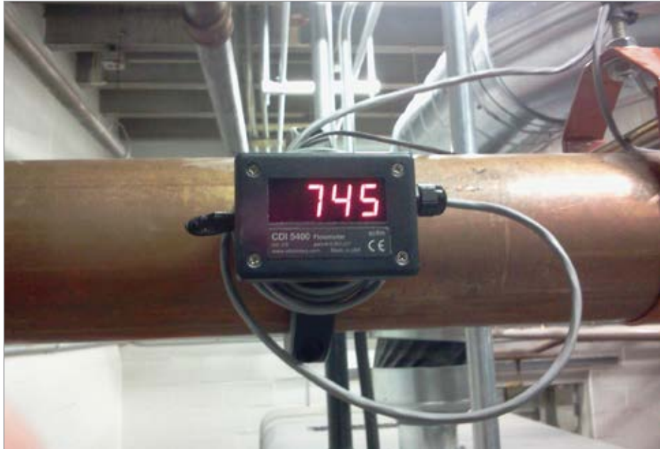
CDI 5400 flow meter installed on a major air distribution line in a lamp manufacturing facility
