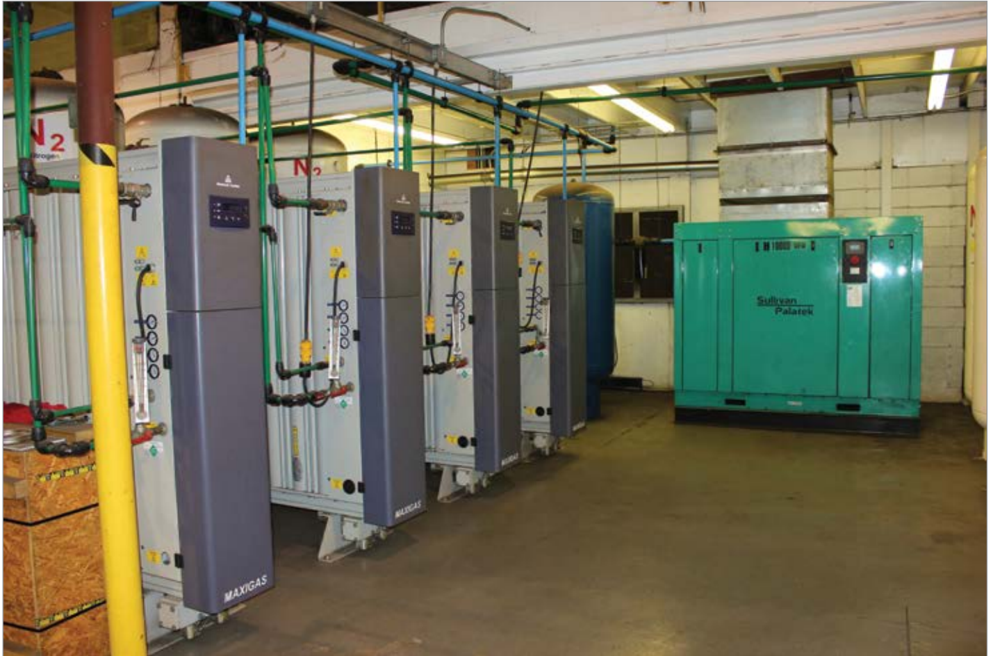
A complete on-site nitrogen generation system.
