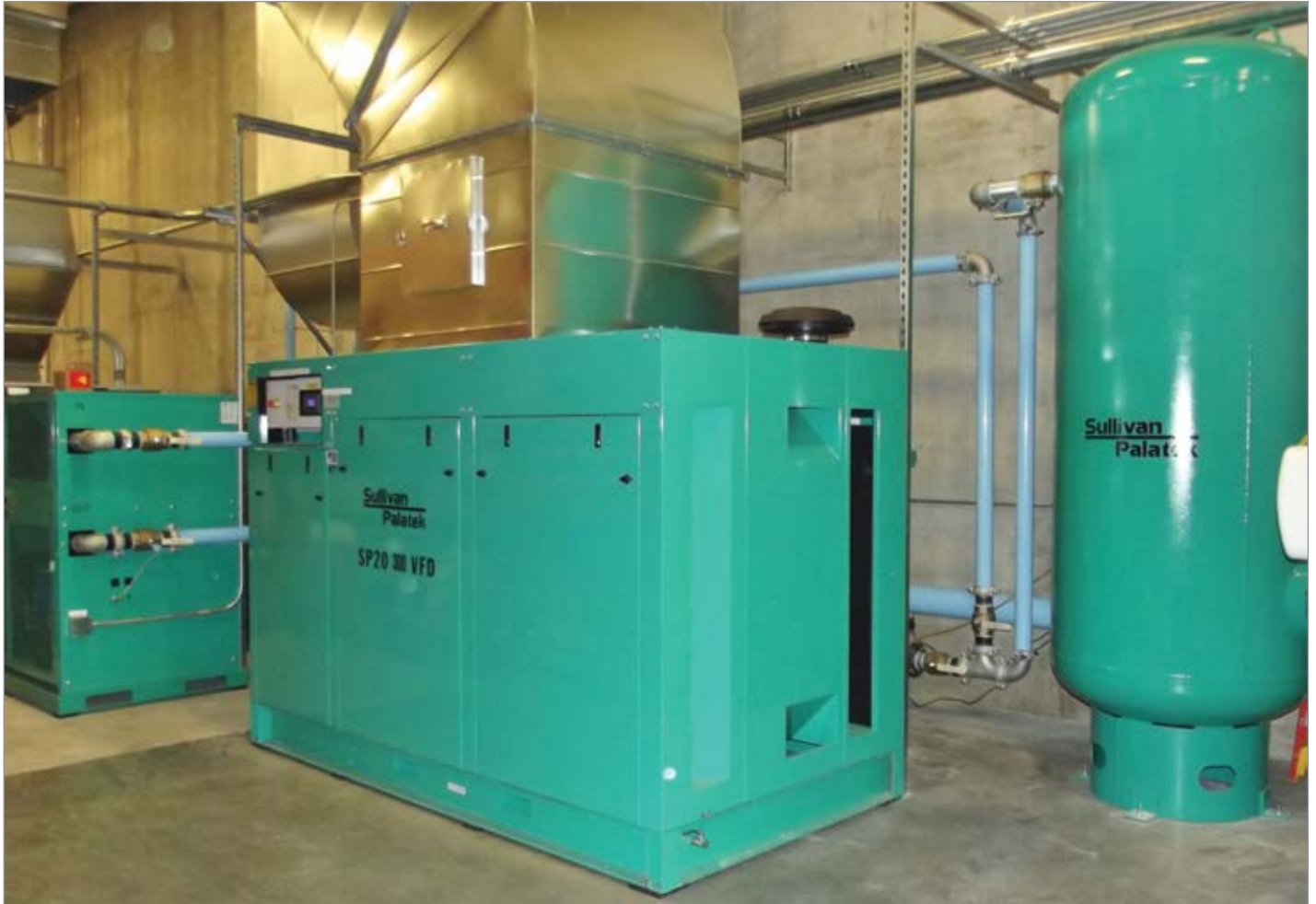
A complete air compressor, air treatment and air storage installation at an industrial plant.
