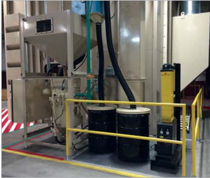
Newly installed sandblast booth with domnick hunter Grade D breathing air system
