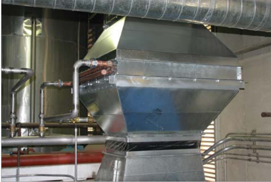
Heat coming off the air-cooled compressors is ducted through finned coils that transfer more than 350,000 BTUs per compressor per hour to preheat the plant's hot water makeup supply.
