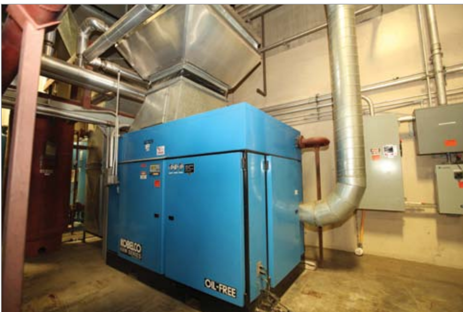
One of four Kobelco KNW series oil-free screw compressors at Nestlé's ice cream factory. Note the air-to-water heat exchanger in the ductwork above.
