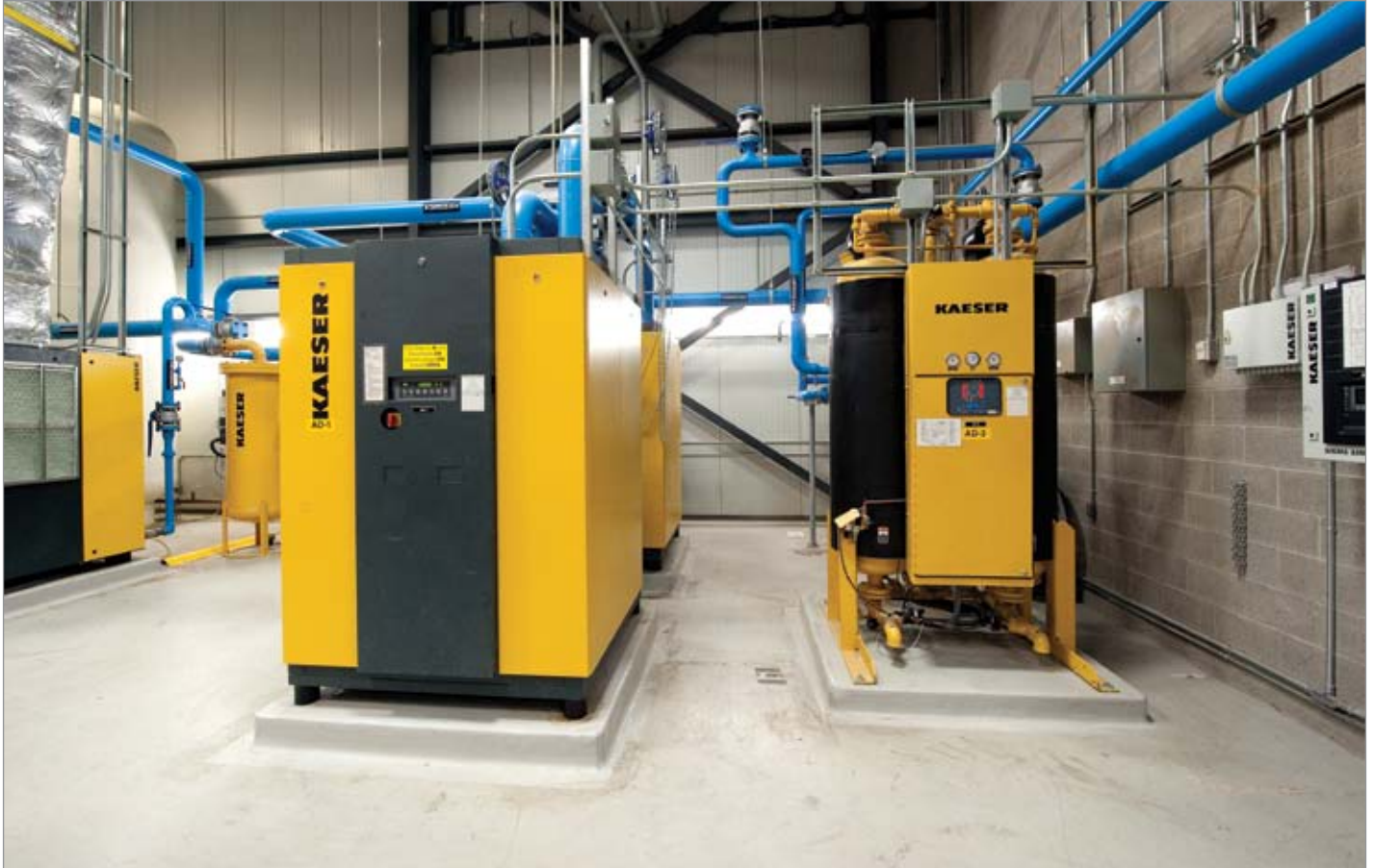
All compressors are controlled, within a narrow pressure band, by a sophisticated sequencing control system and the accurate regulation of the VSD compressors.
