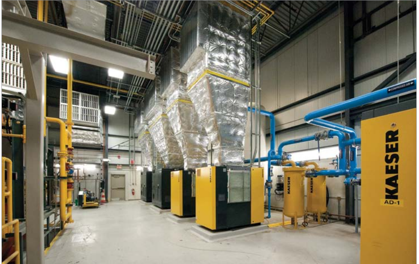
Heat from the new air compressors is recovered in the compressor area.
