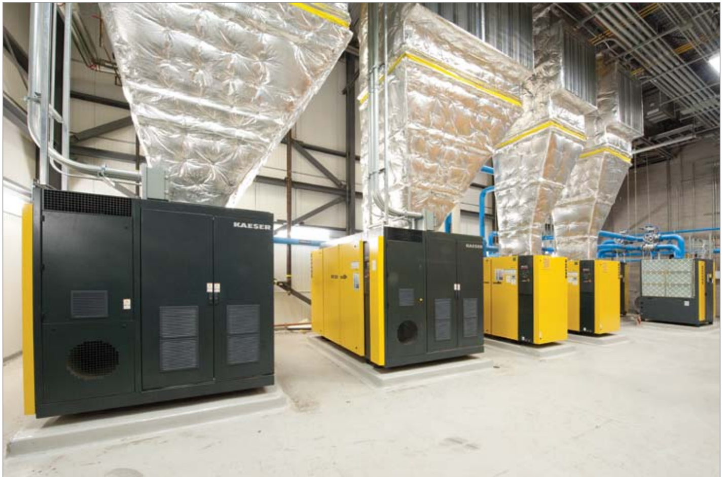
The new system uses four rotary screw compressors and two booster compressors.
