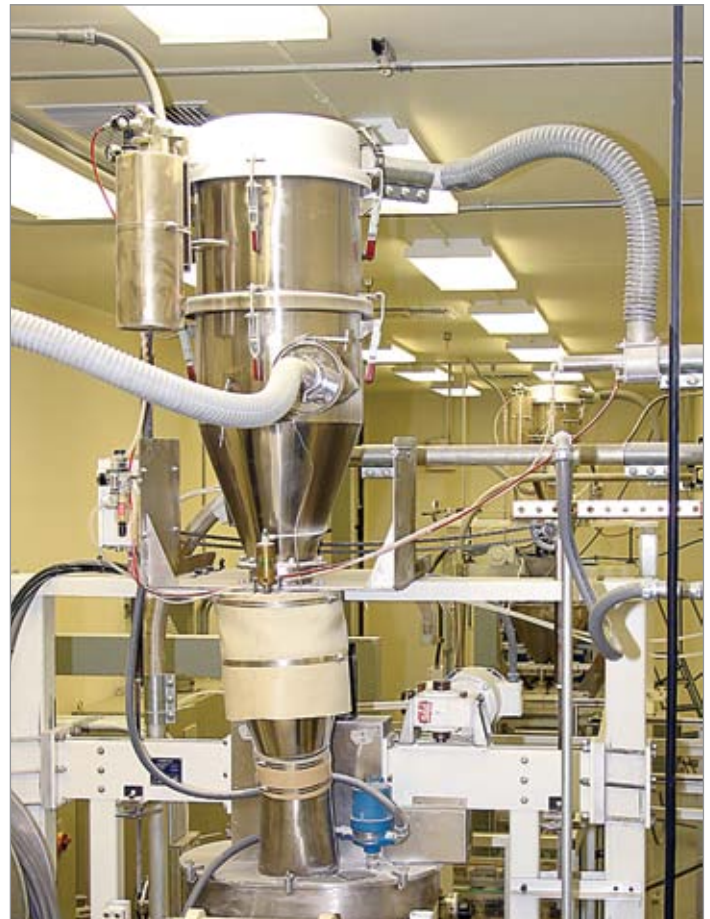
Vacuum conveying systems are adapted according to the level of automation a manufacturer desires and the amount of equipment involved.
