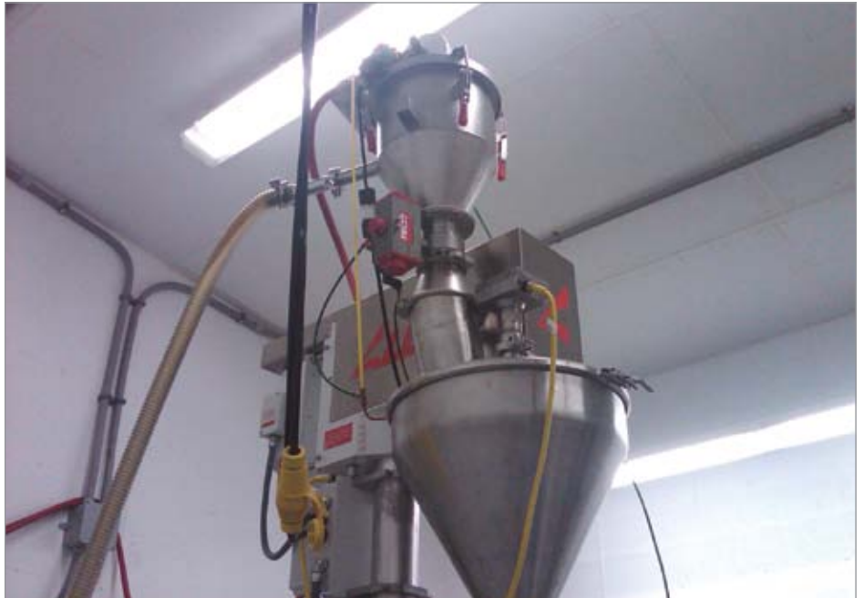
VAC-U-MAX custom pneumatic conveying system above filling machine at Nutriom plant.
