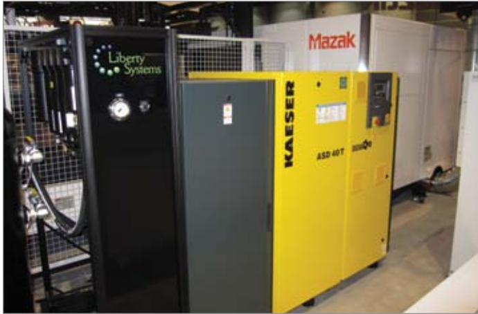
The Mazak Laser Machine Assist Gas Supply System with a Kaeser ASD Series rotary screw compressor.
