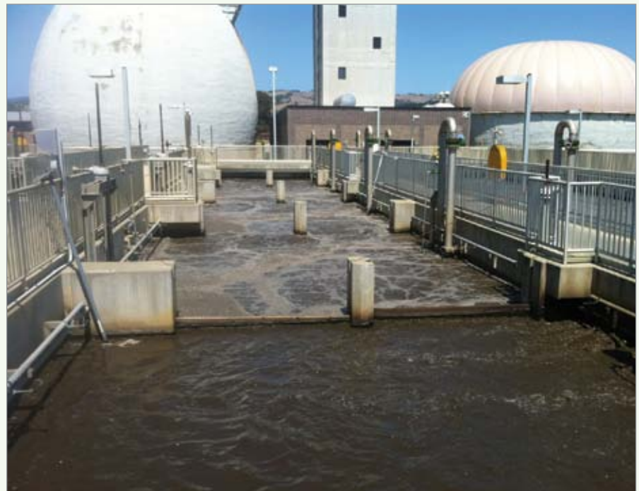
Aeration Basins at NAPA Sanitation District
