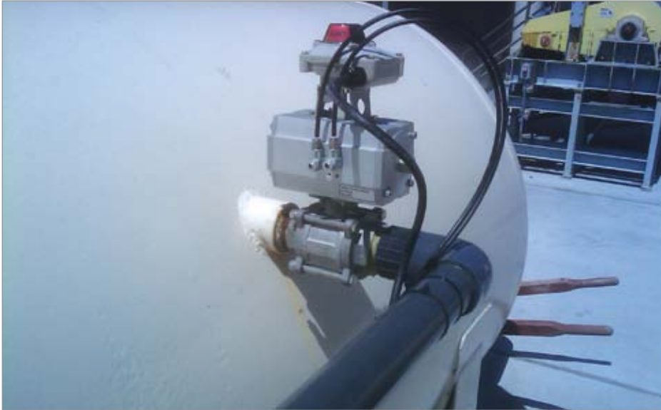
Festo process valve, actuator, and limit switch assembly.
