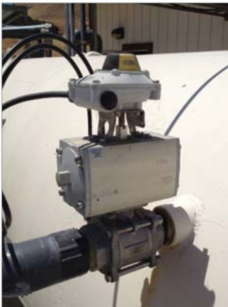
Figure 1. Close up of Festo Process valve, actuator, and limit switch assembly.
