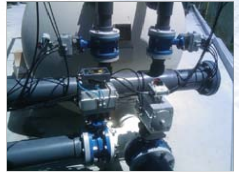
Figure 2. Top, left to right backwash supply valve, effluent discharge valve, and backwash discharge valve.
