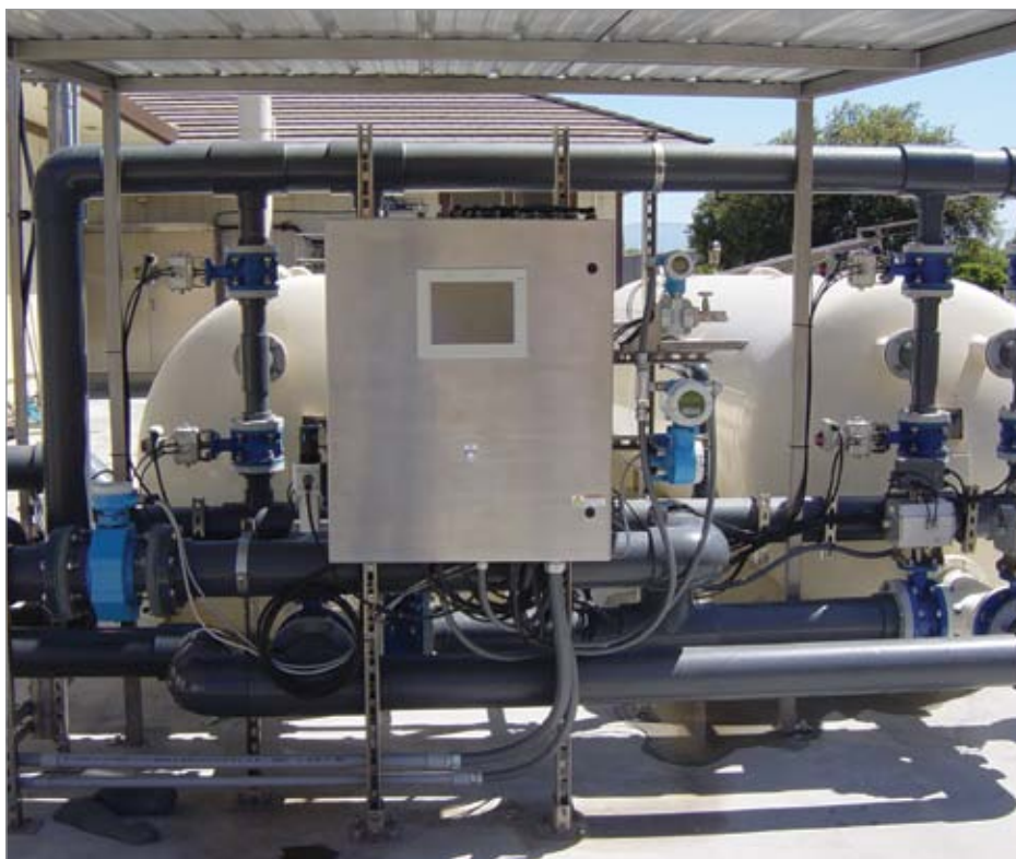
Figure 4. Plant Overview. Control Panel, Process Valve Assy. & Filter Cells.
