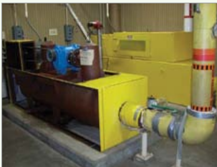
Replaced Positive Displacement Blower
