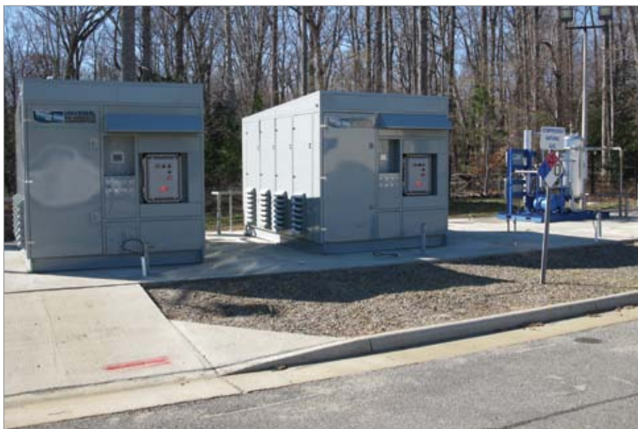
Twin 125 horsepower compressor packages with inlet desiccant dryer for large time-fill NGV Refueling System for Refueling Transit Buses.
