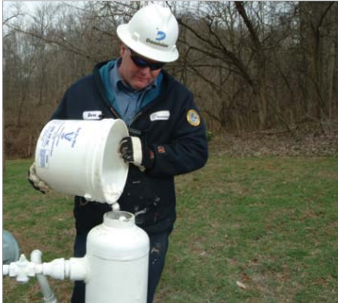
An 8" diameter deliquescent gas dryer is filled with GasDry Max desiccant at a farm tap in West Virginia. The owner of the well must dry the gas in order to meet a sales gas moisture specification.
