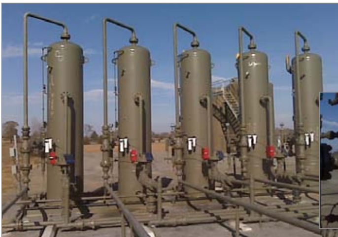
Instrument gas dryers, with 1 Micron Particulate Prefilters, protect valves on production separators.
