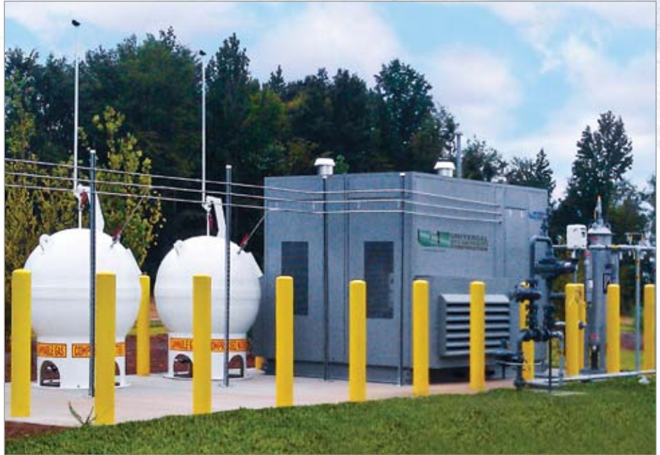
Compression, storage and drying equipment supplying CNG fuel for a public access station.
