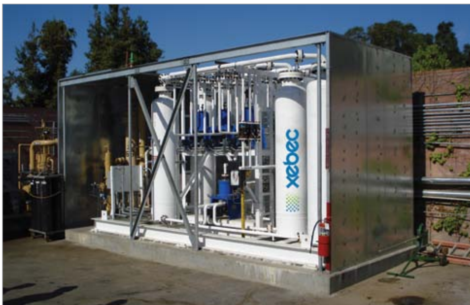
The Xepec compact M-3100 fast-cycle PSA system was the perfect solution to dehydrate field gas at a Southern California oil field.
