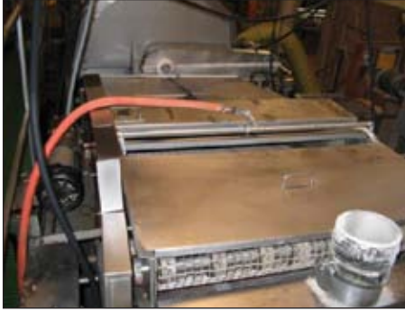
Compressed air pressure dewpoints must be below -15 °F (-26 °C) to inhibit the growth of fungi and microorganisms in the piping system.
